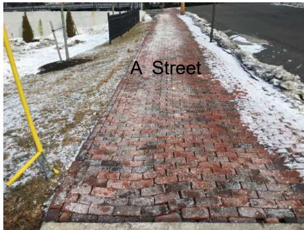
Photo 4 - Uneven settlement along sidewalk.
