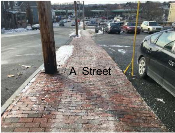
Photo 1 - Uneven settlement along sidewalk.
