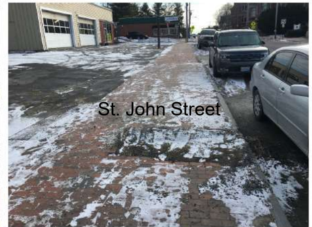
Photo 6 - Unrepaired sidewalk section from utility trenching.
