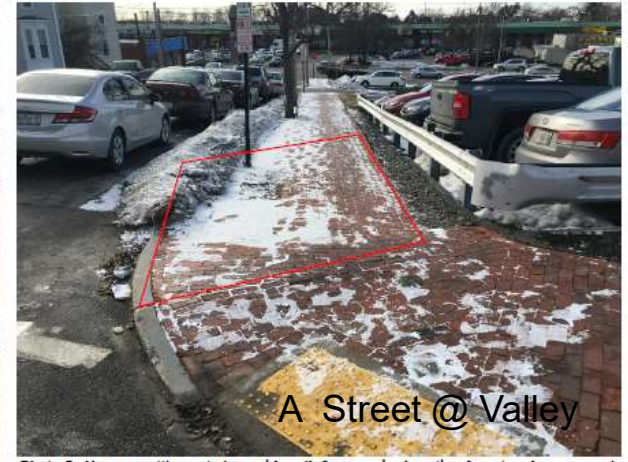
Photo 5 - Uneven settlement along sidewalk & unrepaired section from tree box removal.
