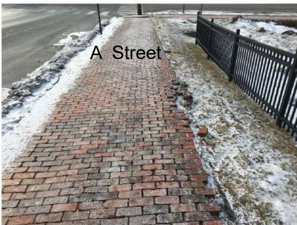
Photo 2 - Uneven settlement along sidewalk.
