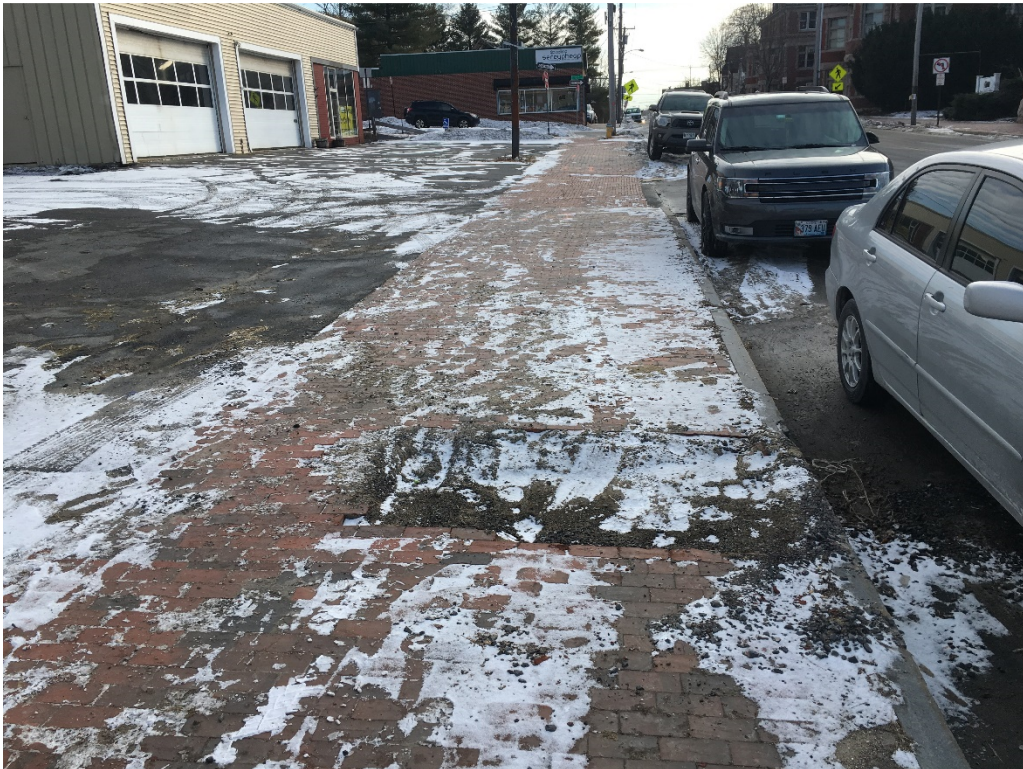
Photo 6- Unrepaired sidewalk section from utility trenching.
