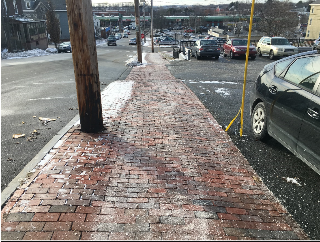
Photo 1 – Uneven settlement along sidewalk.
