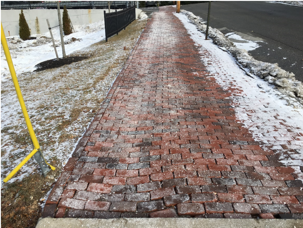
Photo 4 - Uneven settlement along sidewalk.
