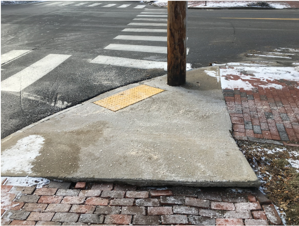
Photo 3 - Uneven settlement along sidewalk adjacent to ADA Ramp.
