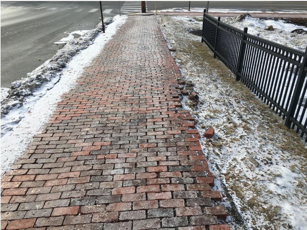
Photo 2 - Uneven settlement along sidewalk.
