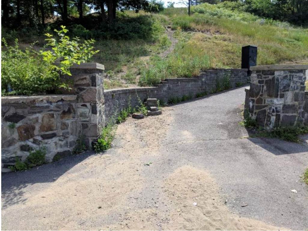
Photo 1: Erosion from retaining wall
