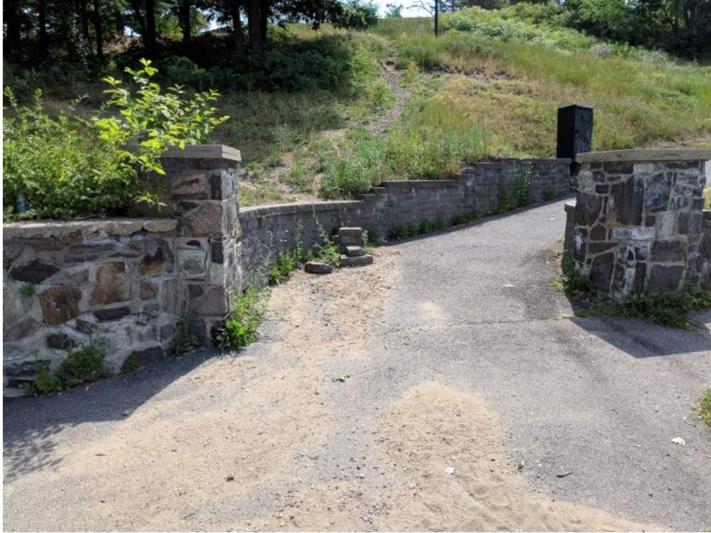
Photo 1: Erosion from retaining wall
