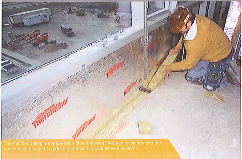
Thermafiber Safing and FireSpan™ insulation provide the critical components of the perimeter fire containment system in the 111 South Wacker Building in Chicago, IL. Thermafiber insulation also contributed to the building's LEED® Gold Rating.
