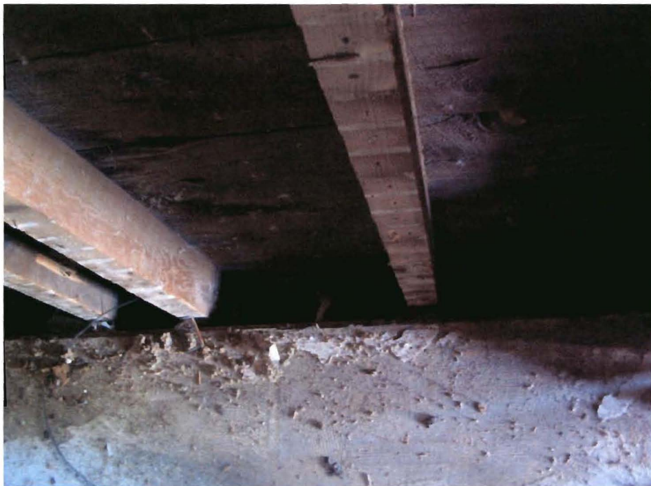
Studs at floor level, no fire blocking
