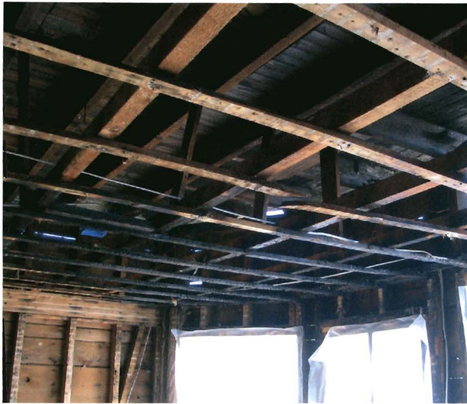
Fire damage at 2 nd floor ceiling
