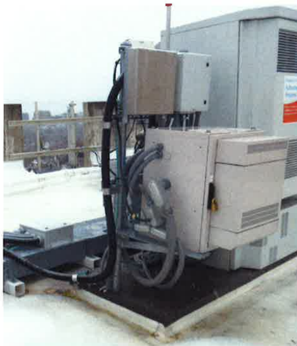
Photo 4: Sample photo illustrating the existing Purcell cabinet on existing H-Frame (to be reinforced).
