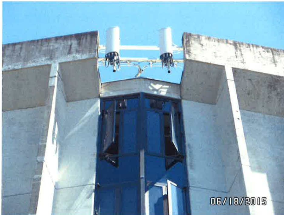
Photo 2: Sample photo illustrating the existing antennas.
