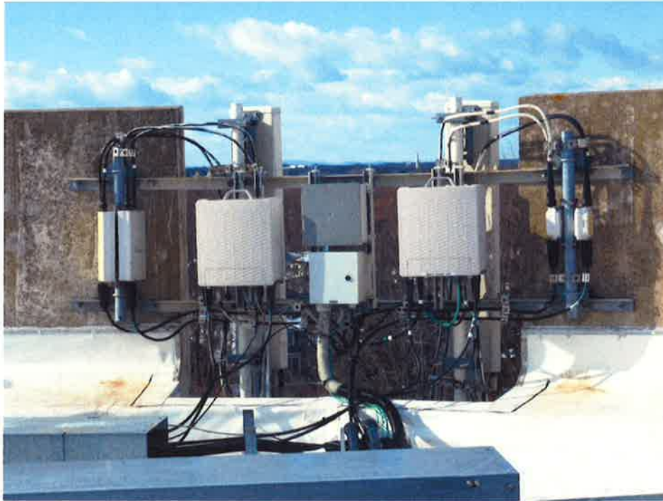
Photo 3: Sample photo illustrating the existing antennas.
