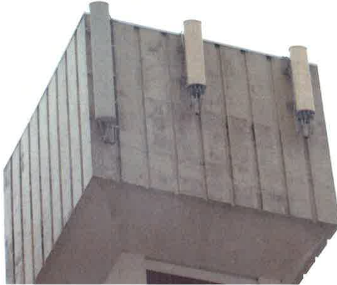
Photo 1: Sample photo illustrating the existing antennas.
