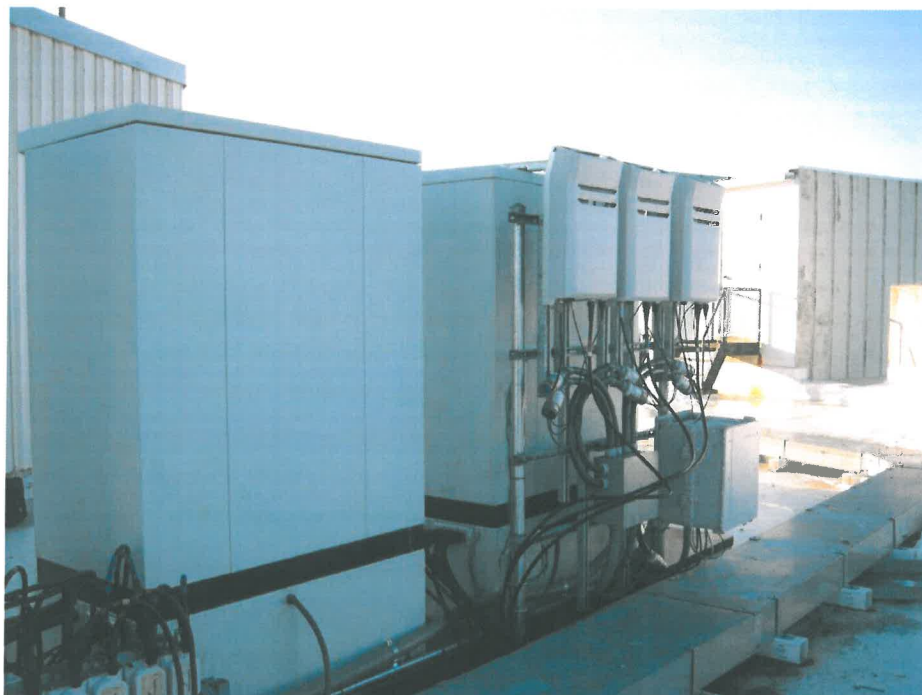
Photo 5: Sample photo illustrating the existing equipment.
