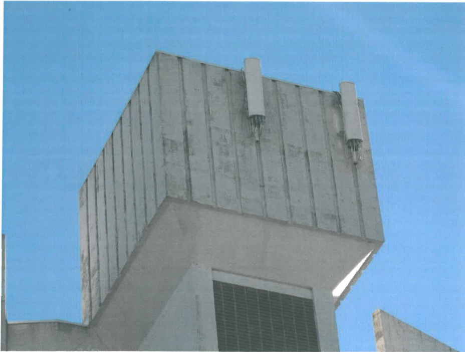
Photo 1: Sample photo illustrating the existing Alpha sector antennas.
