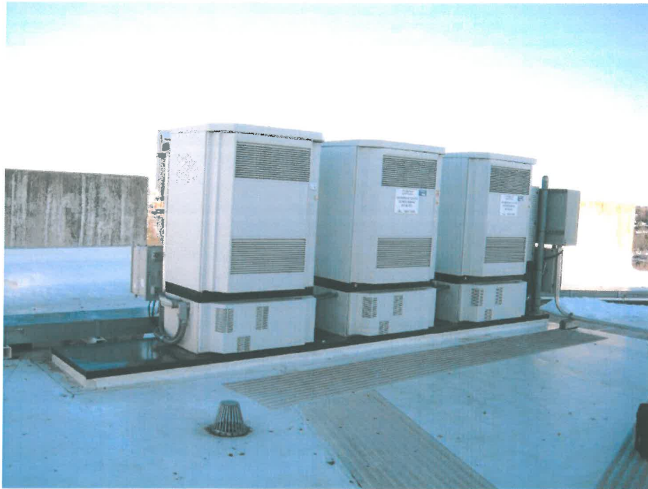
Photo 4: Sample photo illustrating the existing equipment.
