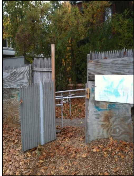
Above:: View looking east to play area entrance from sidewalk leading from parking area to rear building entrance. Fence and gate will be replaced.
