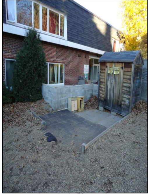
Above:: Existing shed will be reset in same location. Cinder block retaining wall, which houses existing catch basin will remain in place.
