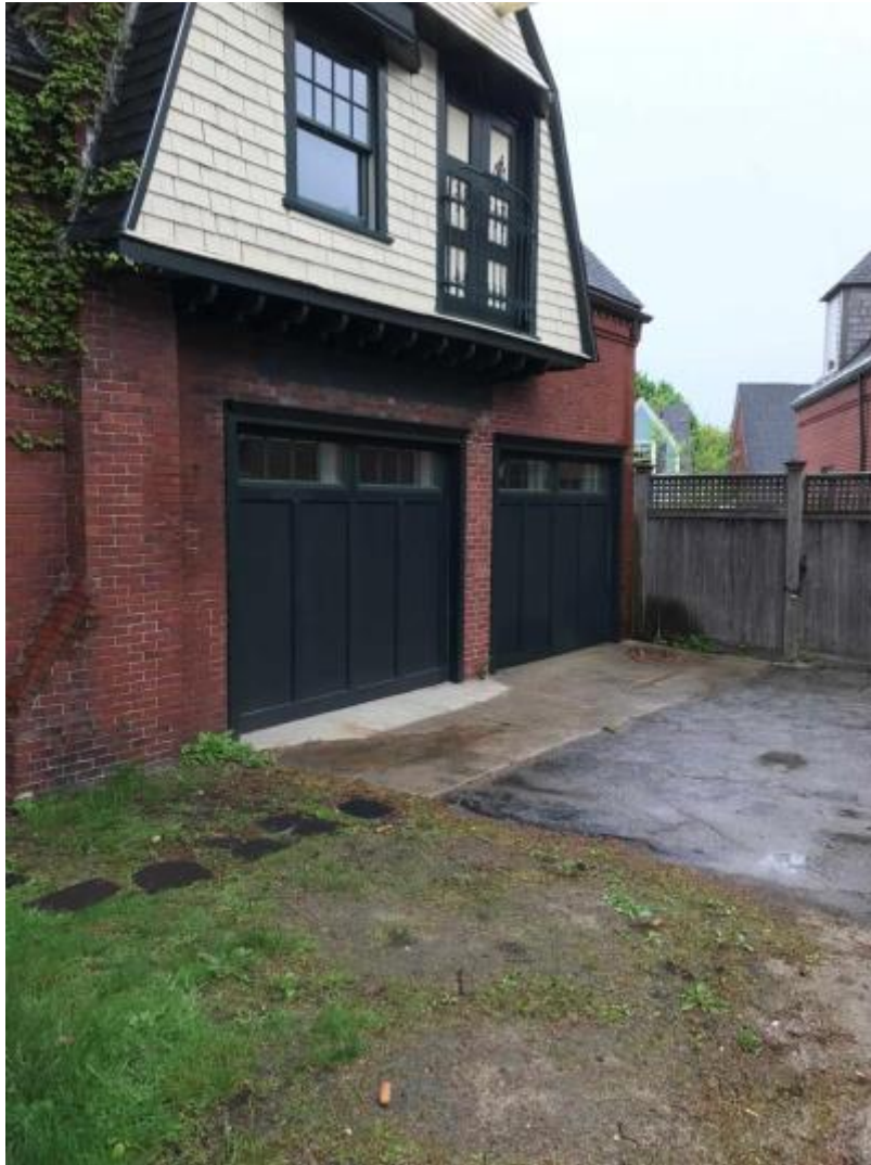
2 IMG_0168 Date Taken: 5/22/2017 Taken By: ANDREW Garage doors previously filled and carry 2 sets each crank windows as shown on drawing.
