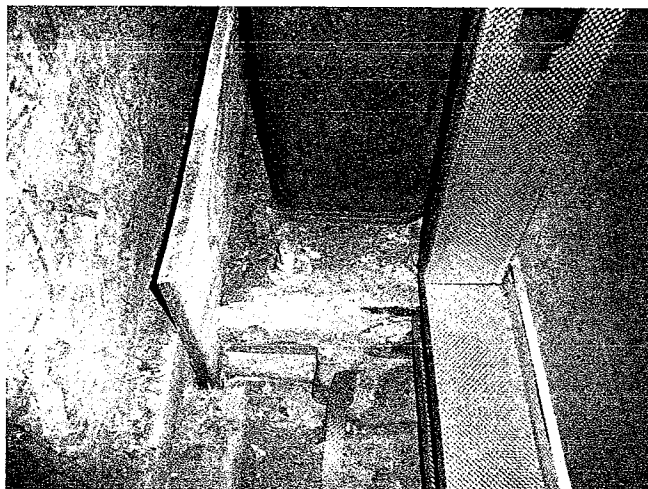
Photo # 2 – Column F/5.8 non- shrink grout below base plate and anchor bolts.
