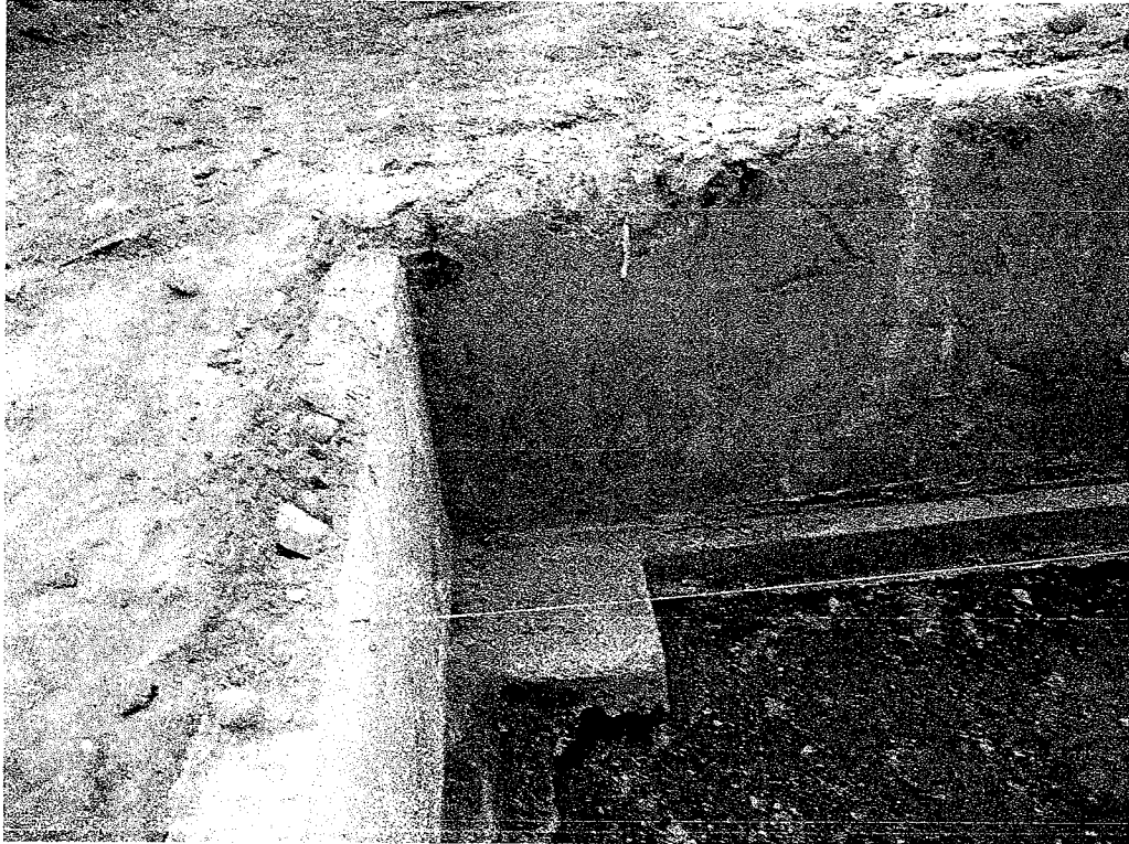
Photo # 3 – View looking north at grade 4.8 - note significant damage to top of existing concrete wall located at grade G.1/4.8 (occurred during demolition).
