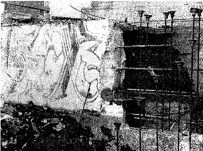
Photo # 5 Spalled Exist. wall @ Rear Sidewalk
