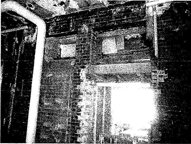
Photo # 1 Lack of Shoring @ 1 st Floor Grid F/3.6
