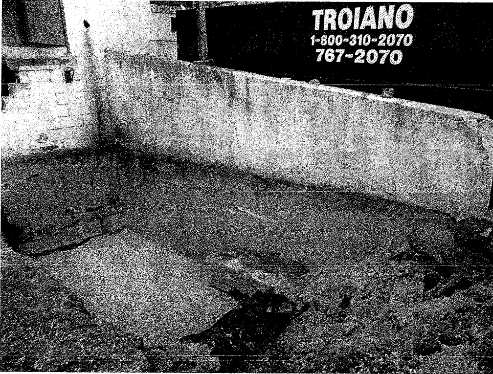
Photo # 1 – Compacted stone at grid G.1/4.2 as recommended by S. W. Cole engineers
