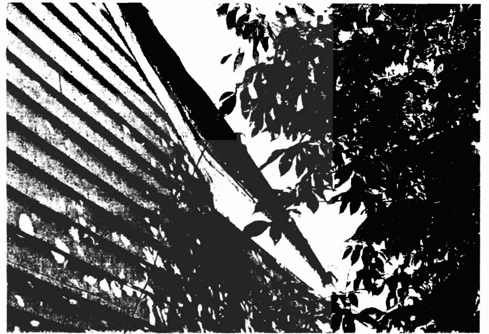
false roof to be removed
