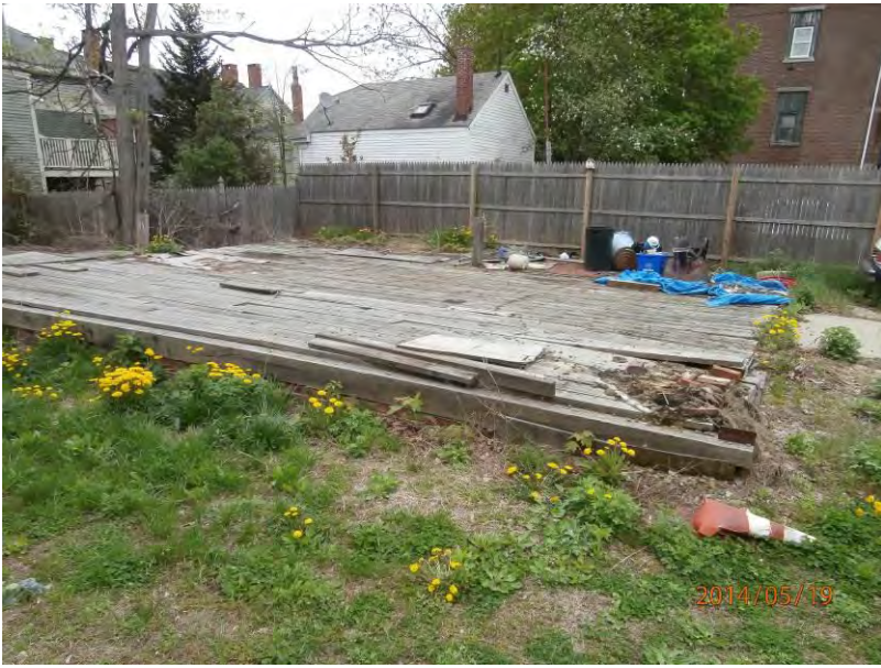
8. Image showing the concrete and wood former barn foundation at the Site, view facing northeast.
