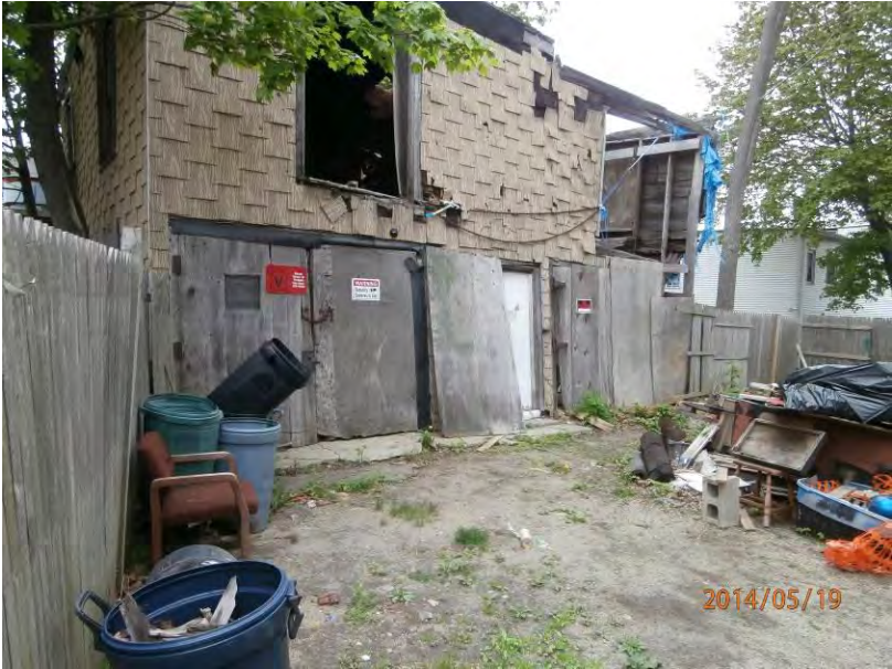
5. Image showing the dilapidated shed/garage, view facing northwest.
