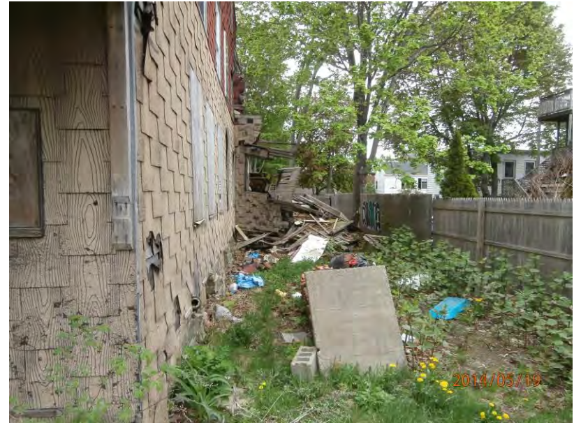
10. Image showing debris behind the residential building.
