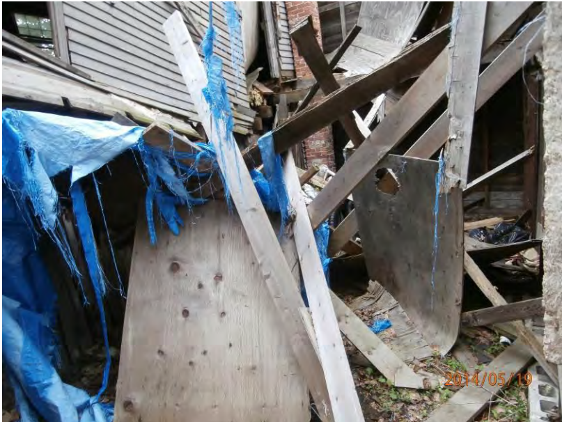
6. Image showing the dilapidated shed/garage.
