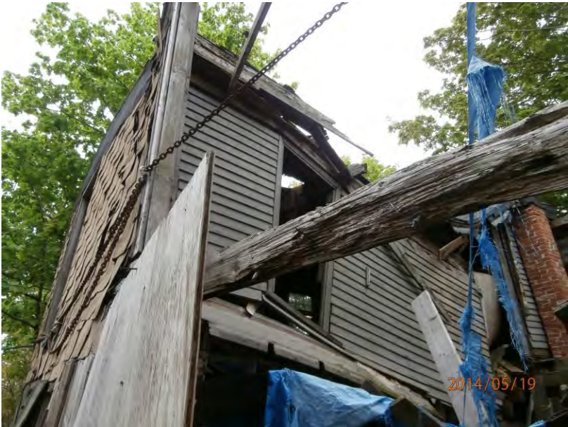
7. Image showing the dilapidated shed/garage.
