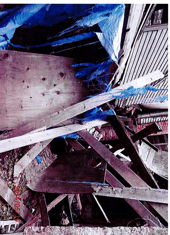
6. Image showing the dilapidated shed/garage.
