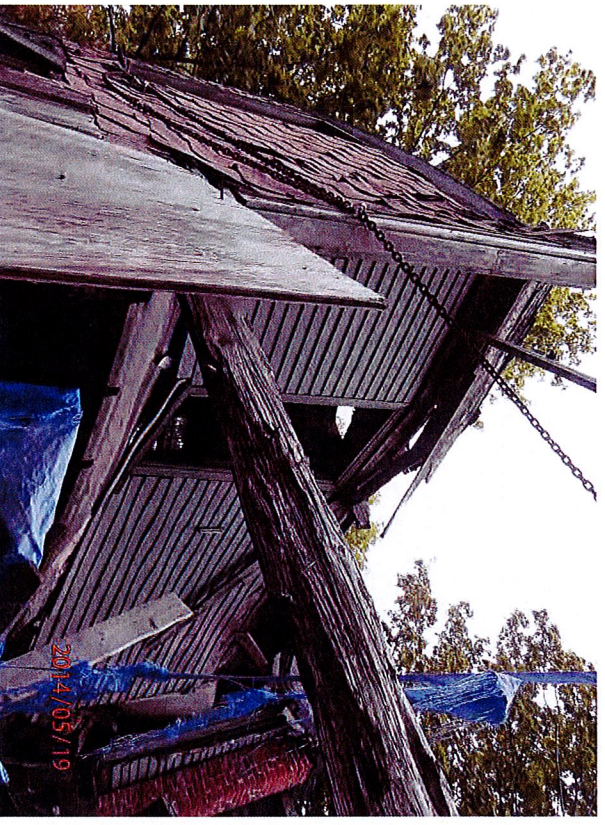
7. Image showing the dilapidated shed/garage.
