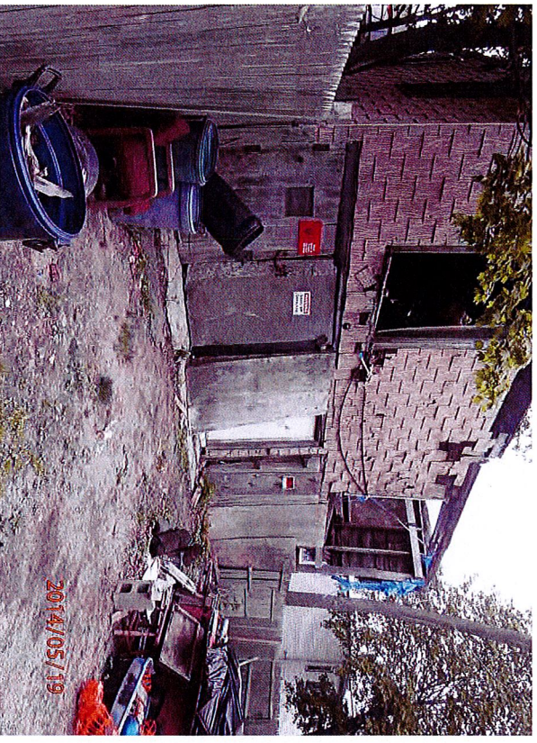
5. Image showing the dilapidated shed/garage, view facing northwest.
