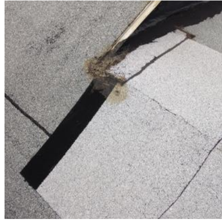
Roof Transition Area to be Repaired
