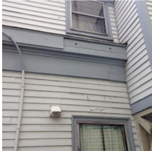
North Face of Residence Missing Fascia Board to be Replaced
