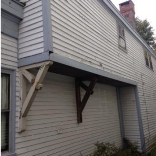
North Face of Residence Corner to be Repaired
