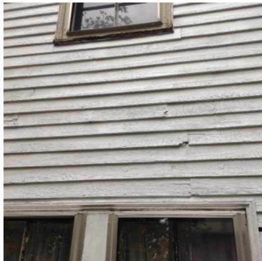
West (Rear) Face of Residence Siding to be Repaired / Replaced / Repainted
