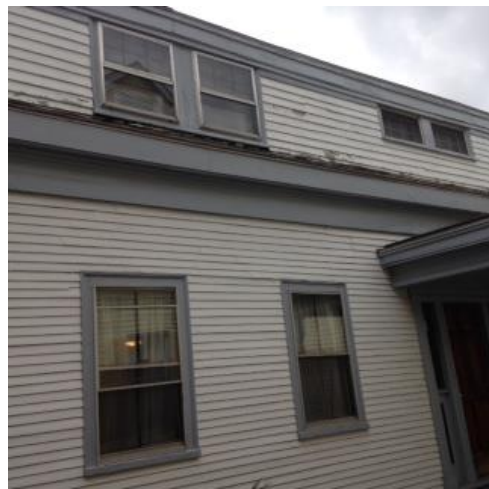
South Face of Residence Misc. Repair Spots along Dormer Line
