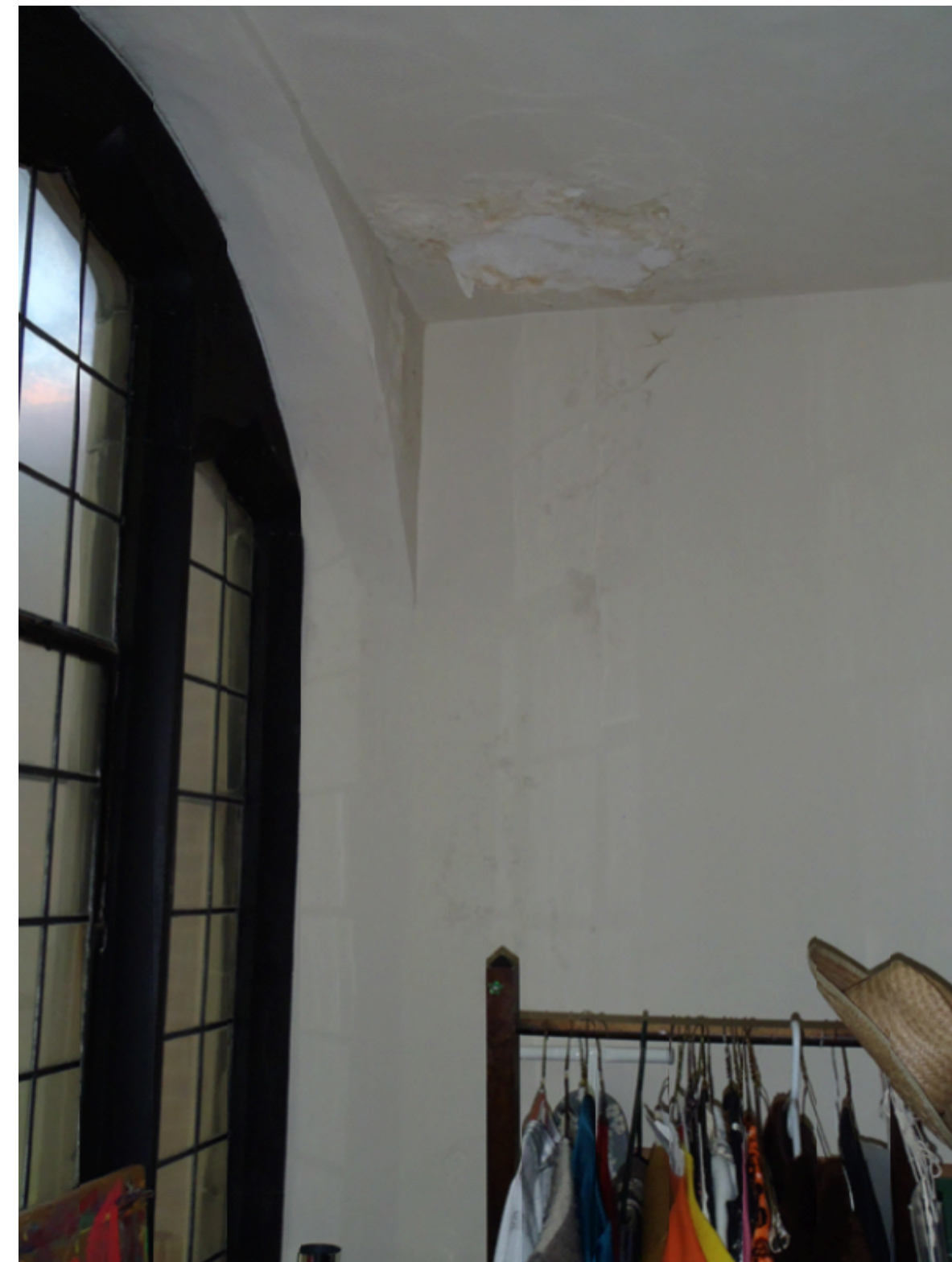
NORTHWEST CEILING/WALL CORNER 50 SF
