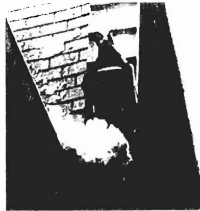
Photo 6: Damaged/Loose Brick at Parapet - West Gable Roof
