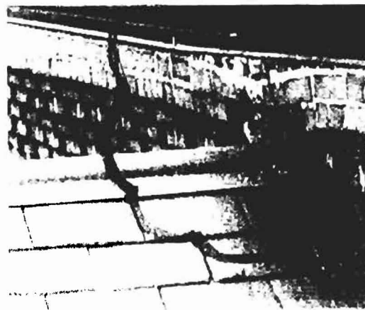
Photo 8: Damaged/Sagging Brick at Office Low Gable Roof
