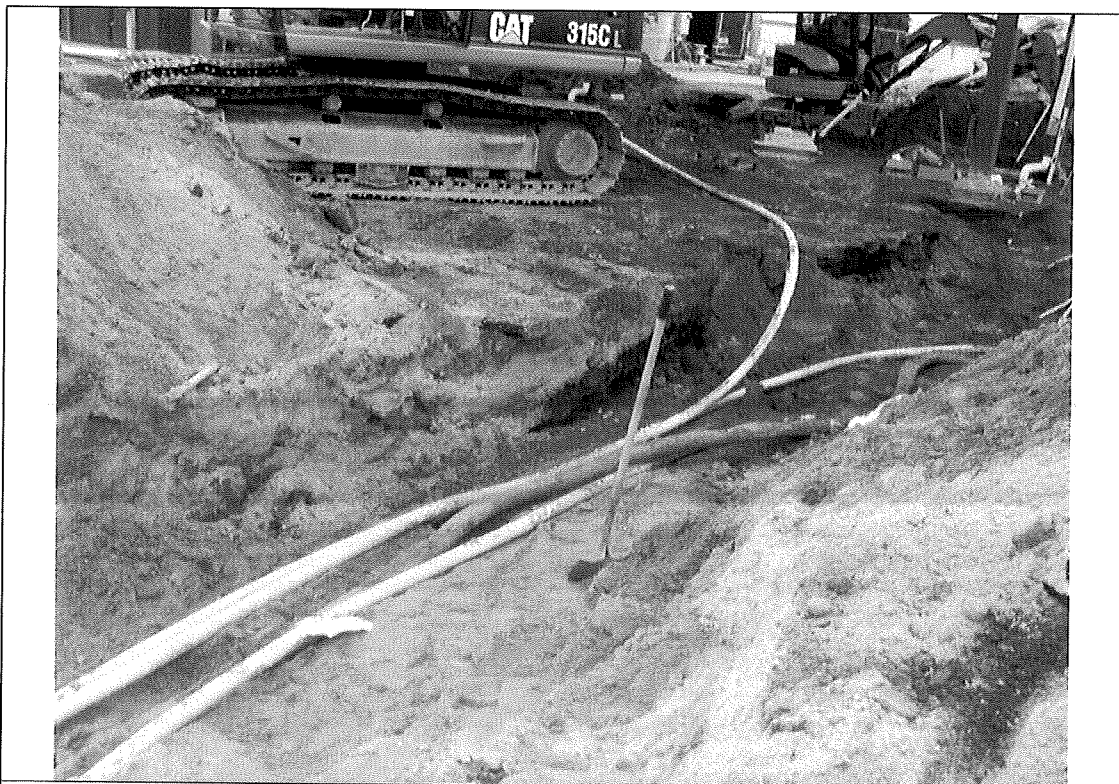
Photograph 4: Product and vapor recovery line to rear canopy, facing south
