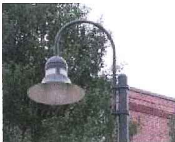
Existing pole & pendant mounted light fixture along Foundry Lane
