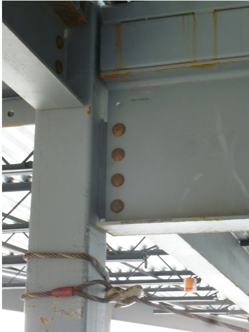
Photo 1: Missing Bolt at W18 to Steel Column 6th Floor Grid K/5
