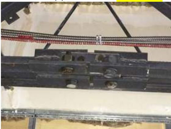
Missing bolt at 5 th floor joist splice. Bolt diameter and ASTM designation to match adjacent bolts. Refer to Vulcraft info. COMPLETED
