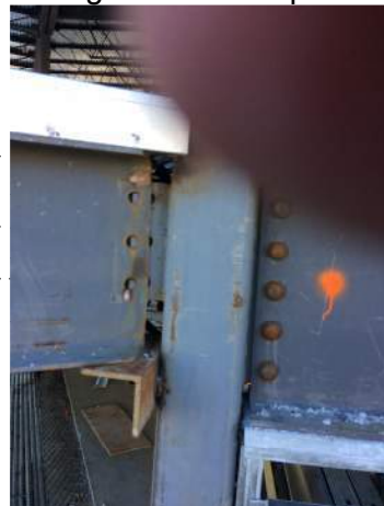
Floor beam @ column A/12 requires welding to connection plate instead of bolts.
