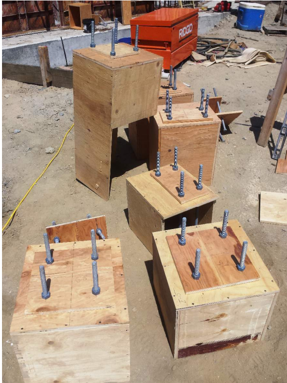
Photo 7) Dropped Pier Bondouts w/ Type AB-1 Anchor Bolts for Piers on A-Line & 17-Line
