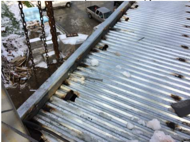
Brick relieving angle and bolts to be cast-in slab. Decking welds to joists underneath.
