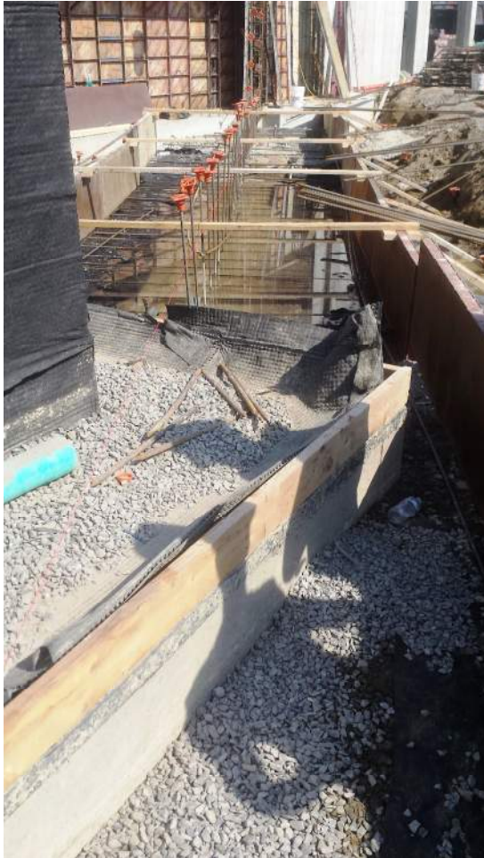
Photo 1) Garage footing protruding into form for building footing near 6.6/B.
