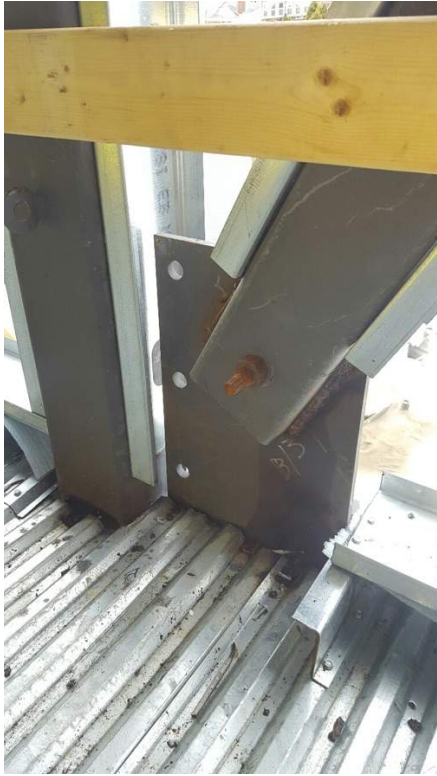
Missing Shear Connection
