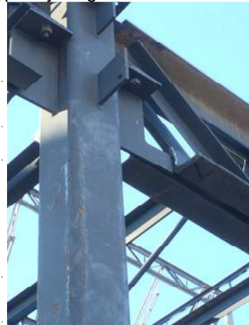
Joist girder chord angle cut to allow installation. Piece to be welded back @ roof joist girders.
