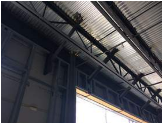
Missing column bracing @ (3) basement tube columns & (1)W18 column. COMPLETED
