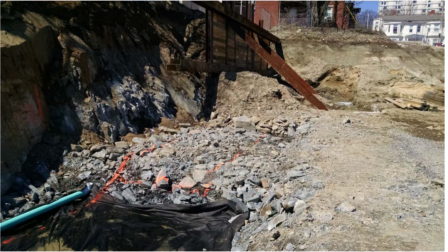
Fractured Rock Fill Placed Along Garage Southern Perimeter Wall Line to be Removed and Replaced
