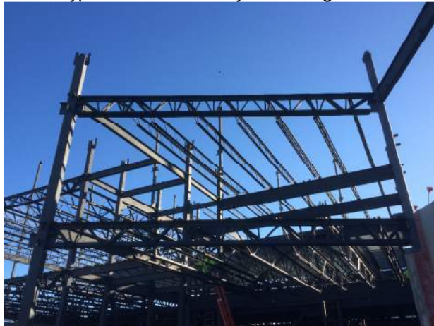
2 nd & 3 rd floor joists & girders progressed from Line 17 (High Street) to line 12.
