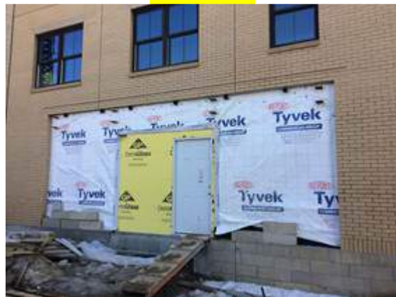
Canopy roof. Let me know when steel is to be erected. WAITING FOR STEEL DELIVERY
