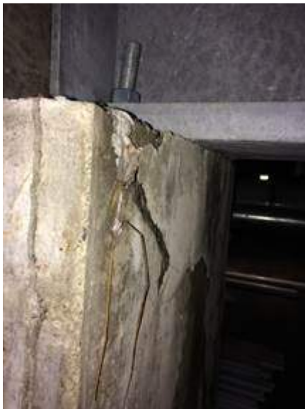
Crack @ left hand side of pier and spalled patch @ front face of pier
