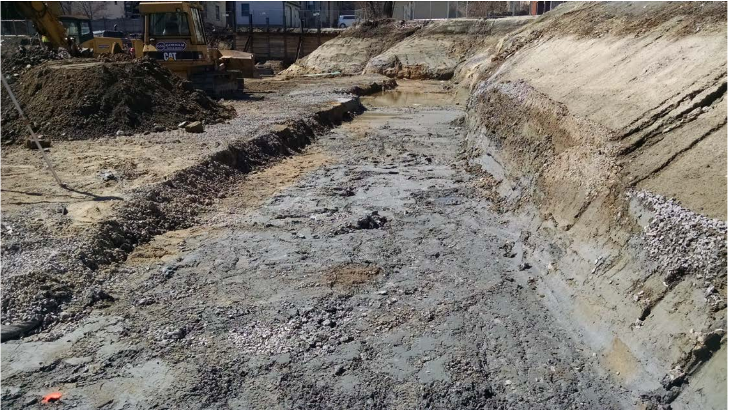
Disturbed Soils Along Garage Northern Perimeter Foundation Wall to be Overexcavated and Replaced
