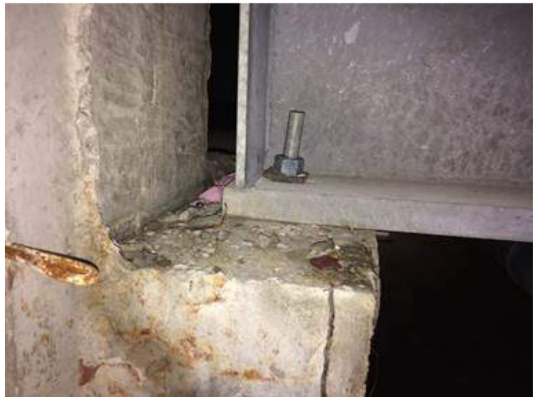
Beam contacts steel bearing plate and edge of concrete.
