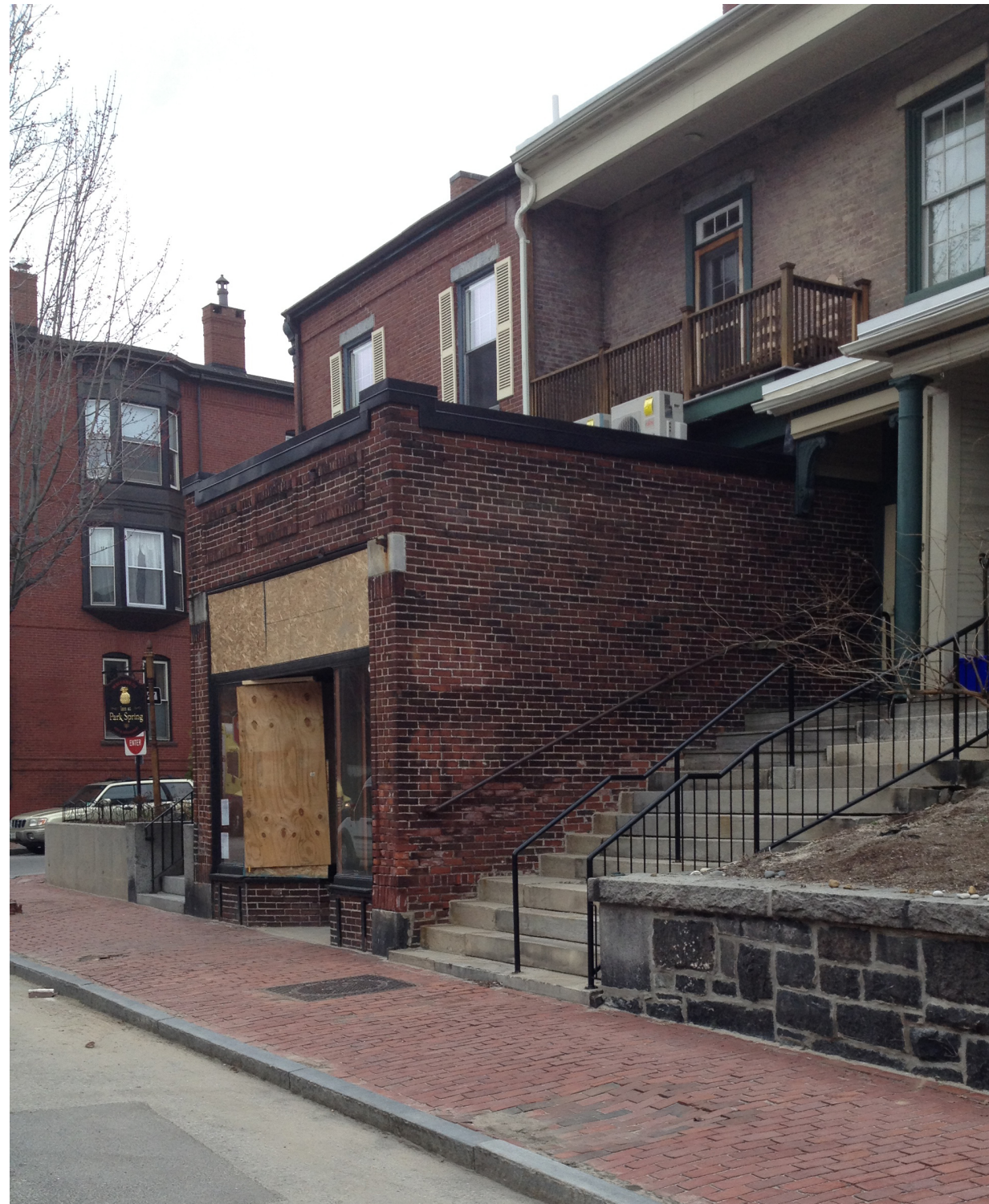
1 Unpainted Heat Pumps
