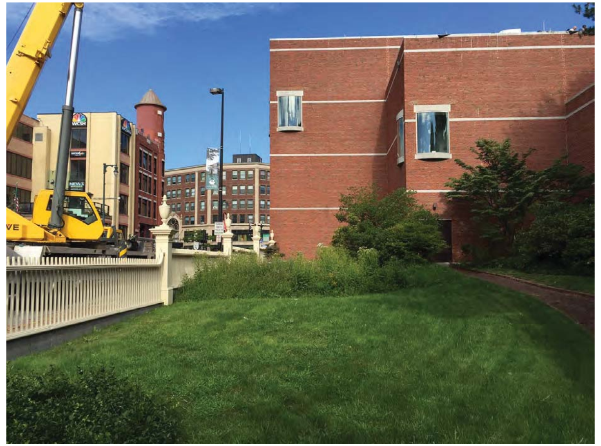
Looking north toward Congress Street. Gate to be inserted in center of second fence panel.
