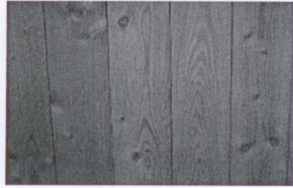
Figure 4. Exposed face of deck specimen 2.
