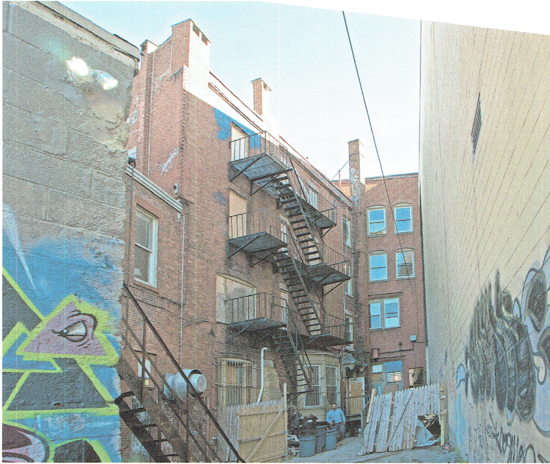
e. Existing Fire Escape (not required given internal stair systems design & not currently to code at this time)
