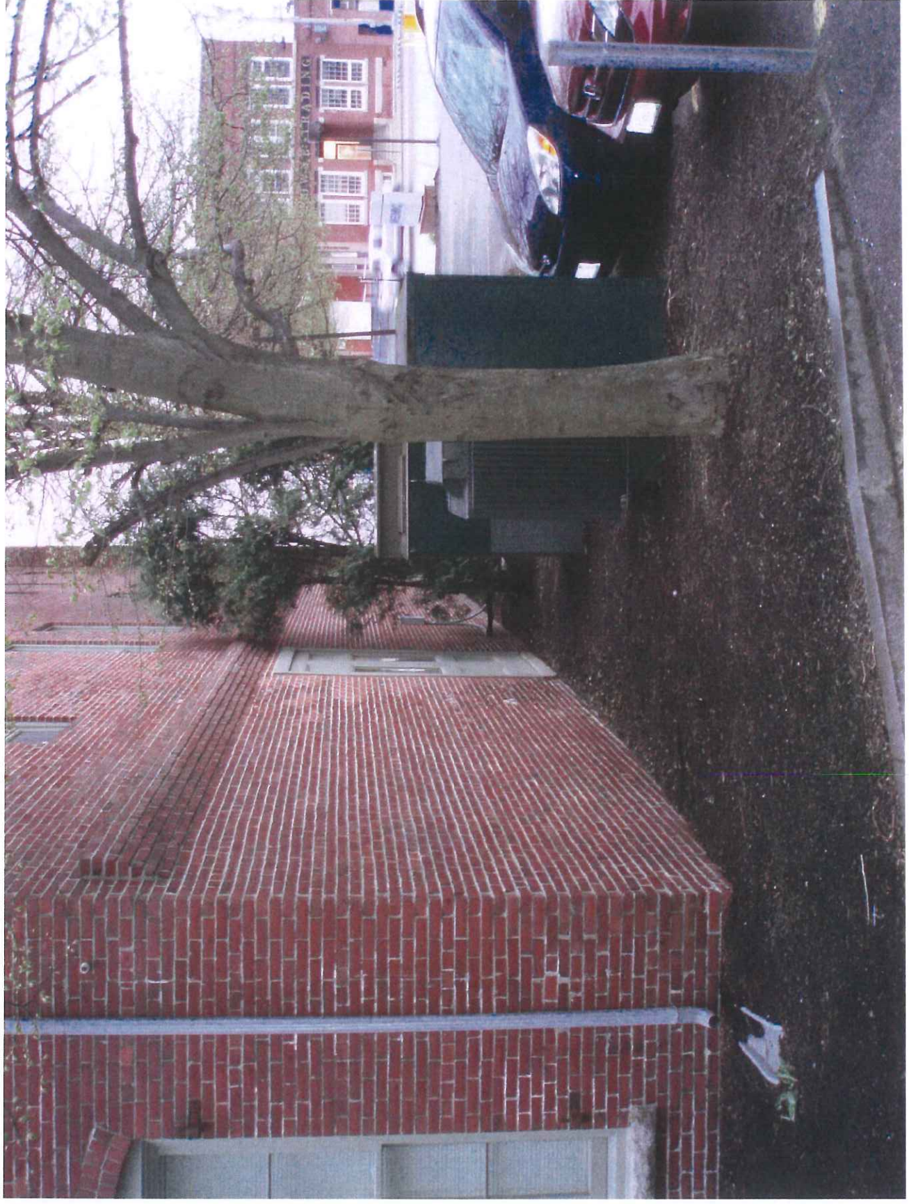
EXISTING TRANSFORMERS (NORTH)
