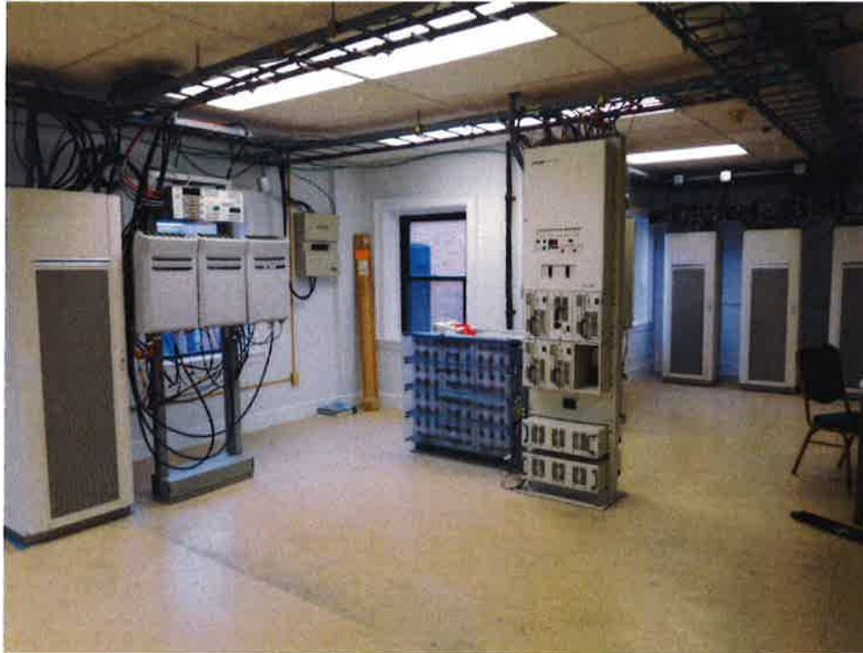
Photo 1: Sample photo illustrating the existing equipment room.
