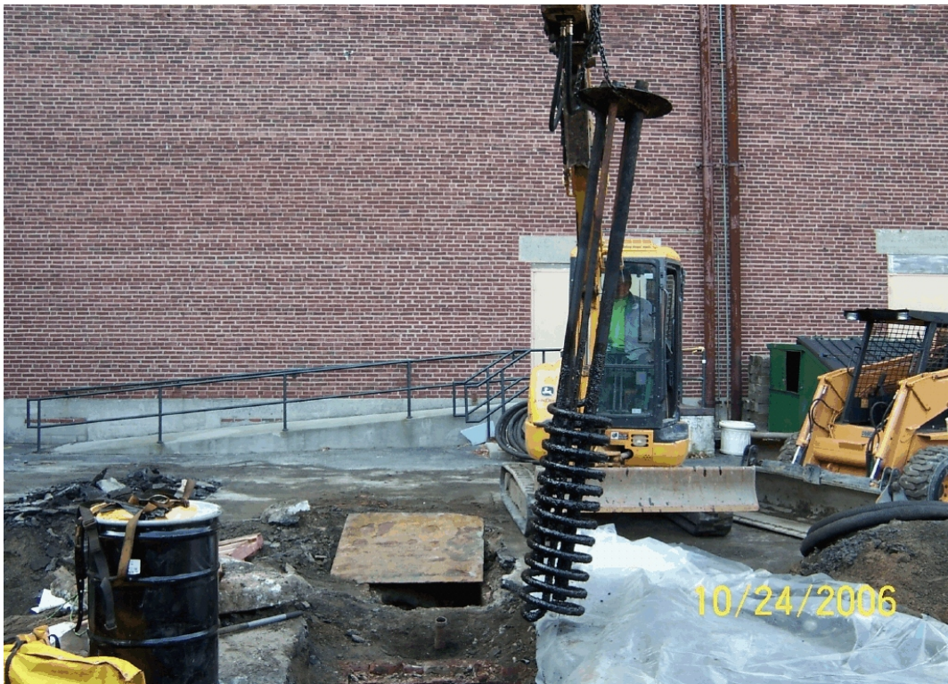
Removal of heat exchanger from Tank. Heat exchanger removed from both tanks.
