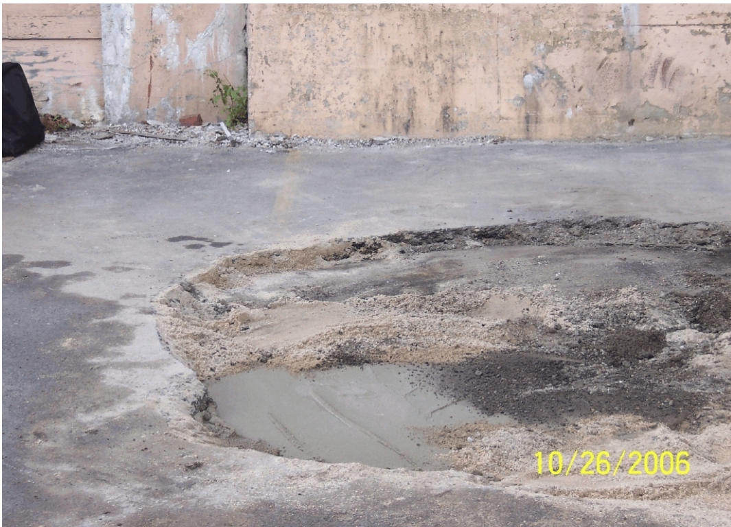
Close-up of slurry exposed in area of accessway in Tank #2.
