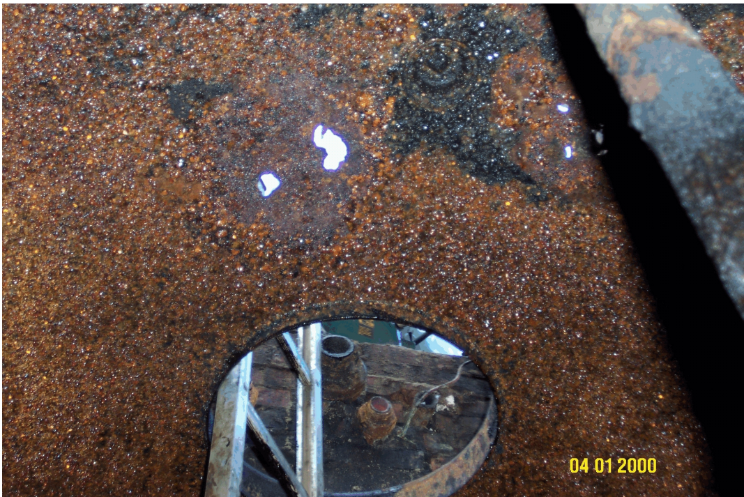
Corrosion on top of Tank #2. Multiple perforations. (Photo date incorrect.)
