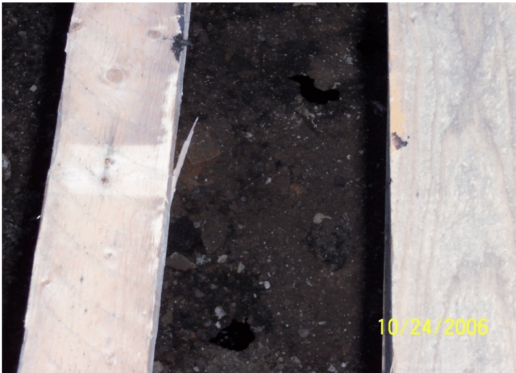
Exterior (top) of Tank #2. Note corrosion holes.
