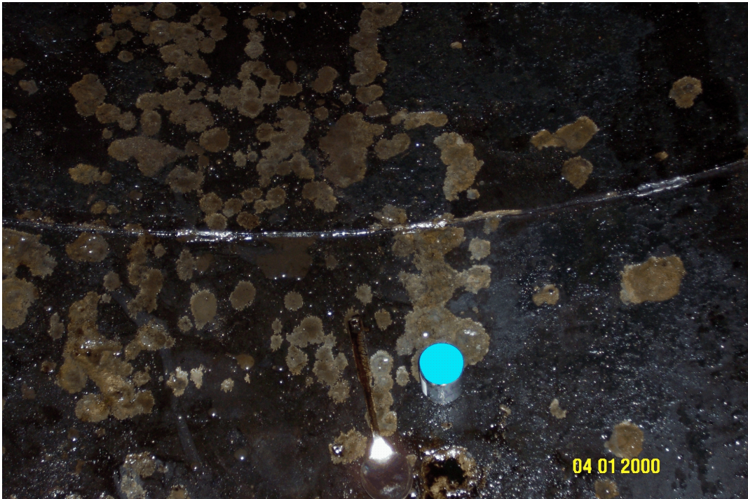
Corrosion on interior of Tank #2. Note large perforation. (Photo date incorrect.)
