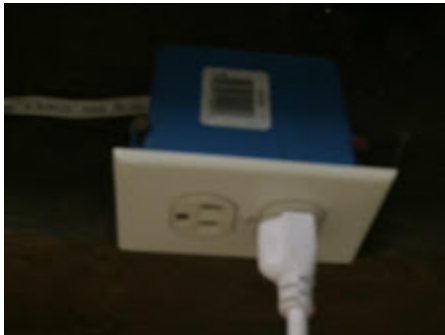
cover plate electric box in laundry room #4.jpg
