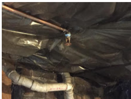
sprinkler head over dryer #2.jpg 32K
