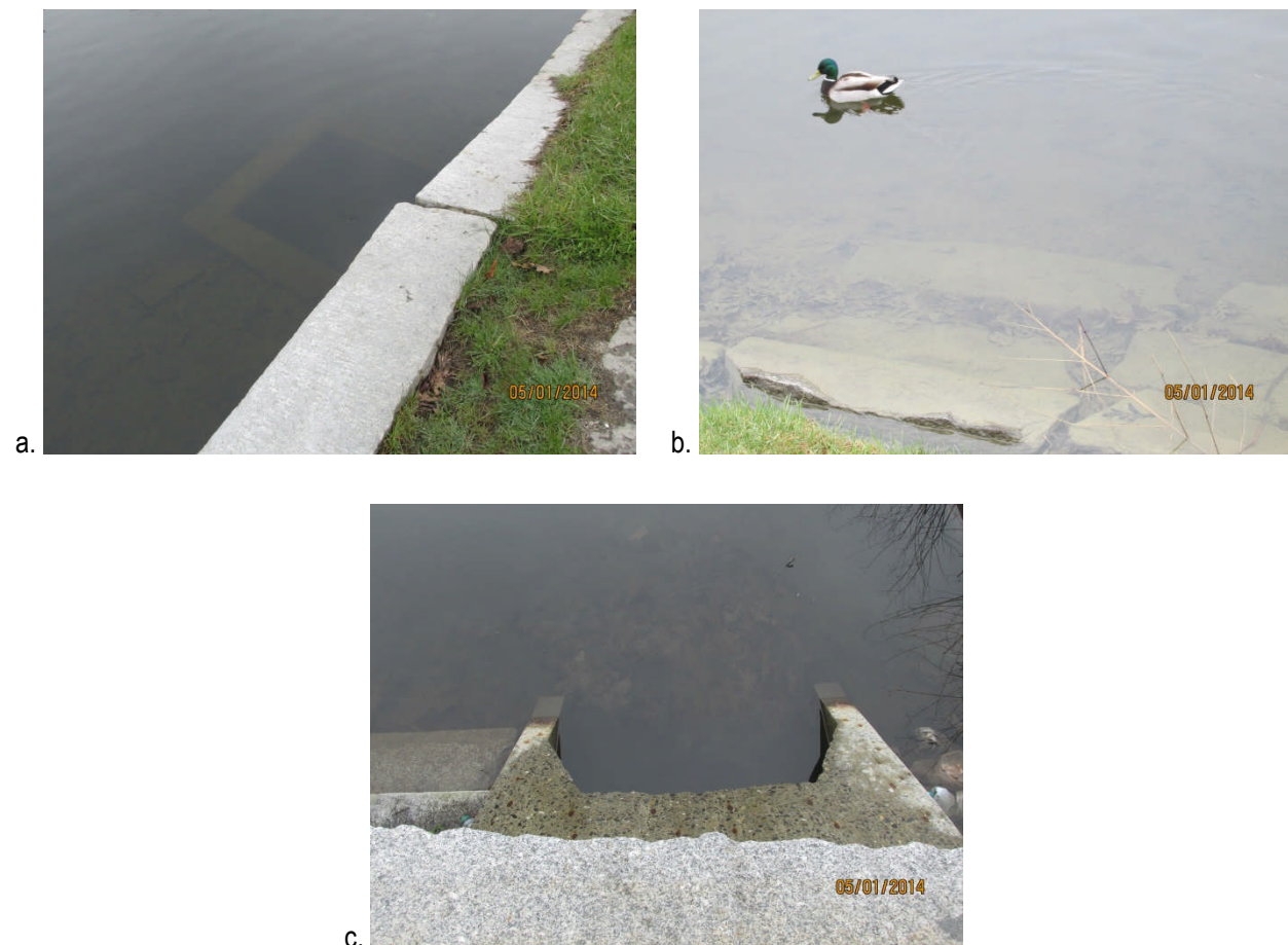
Figure 2-4 Deering Oaks Pond (a) concrete below water surface; (b) granite blocks below water surface at pond edge; and (c) darkened concrete at pond edge.
