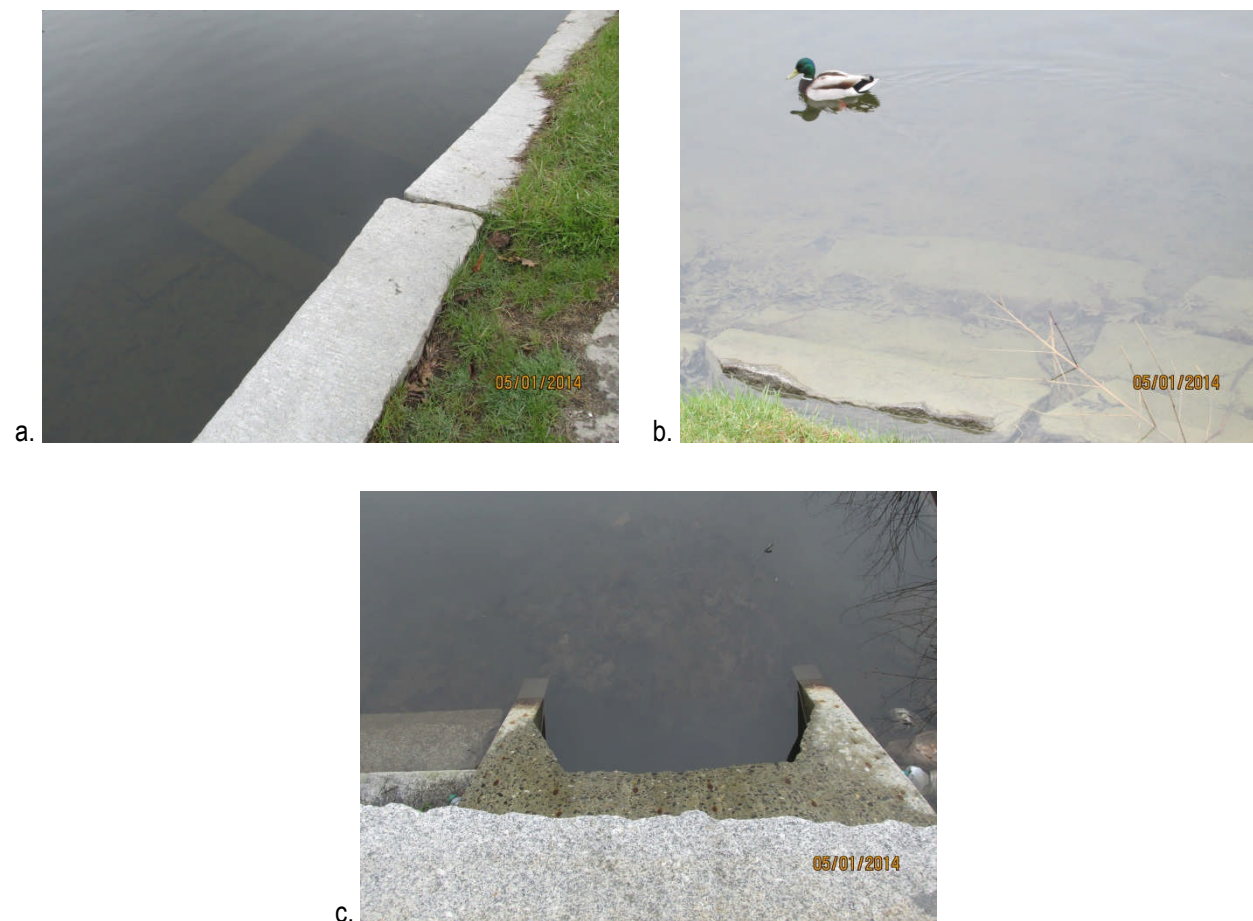
Figure 2-4 Deering Oaks Pond (a) concrete below water surface; (b) granite blocks below water surface at pond edge; and (c) darkened concrete at pond edge.
