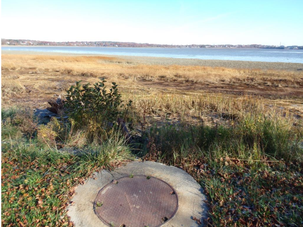
Photo 5: Picture of the existing outfall location at the intersection of Belmeade Road and Baxter Boulevard.
