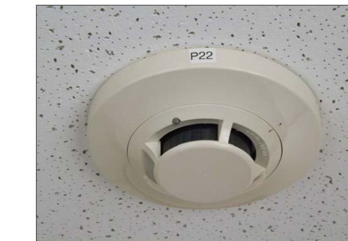
EXISTING DETECTOR AT CORRIDOR AND STAIRS
