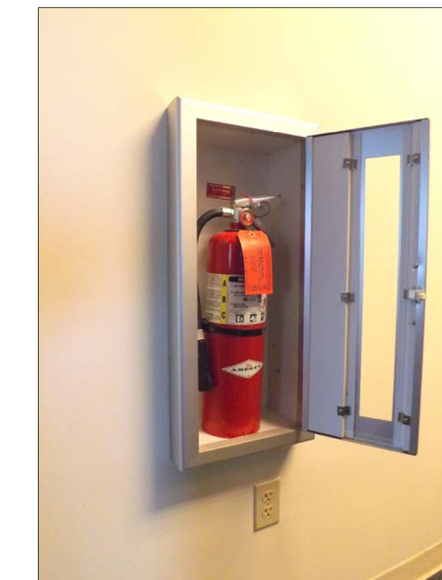
EXISTING FIRE EXTINGUISHER AND CABINET
