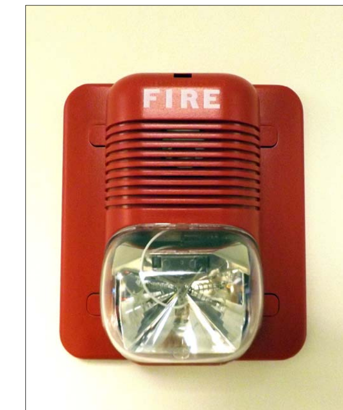
EXISTING HORN AND STROBE
