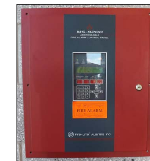
EXISTING PANEL AT 1ST FLOOR LOBBY
