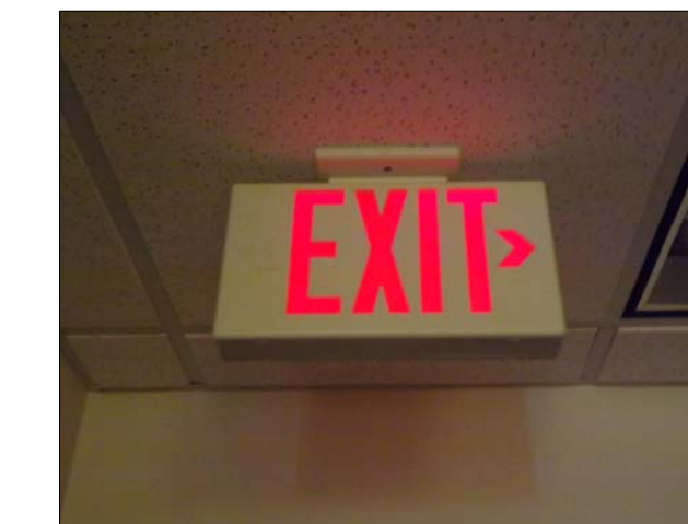
EXISTING EXIT SIGN WITH DIRECTIONAL INDICATION
