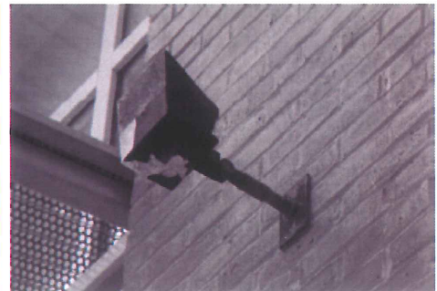
Figure 6: Up-Light to be Replaced
