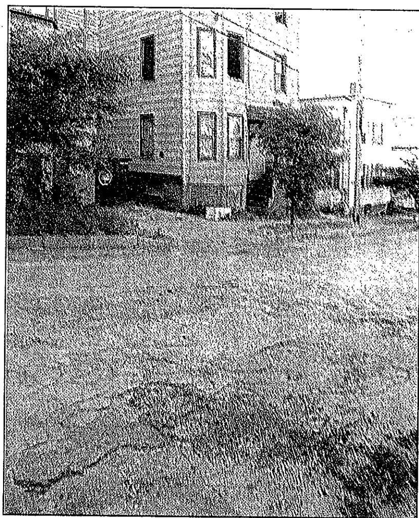
Alder Street's neglected pavement adds to the deterioration of a neighborhood in which there are three abandoned buildings, including two burned-out hulks next to Basil Scott's home.
