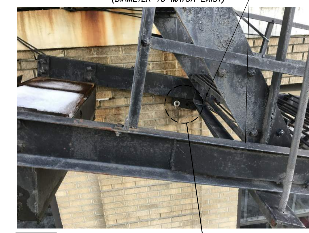
PHOTO 3 UNBOLT & ADD SHIMS AS REQD TO ALLOW FULL MOVEMENT OF SWING SECTION AND REBOLT W/NEW H.D. GALV A307 BOLTS (DIAMETER TO MATCH EXIST) REANCHOR SWING SECTION TO WALL
