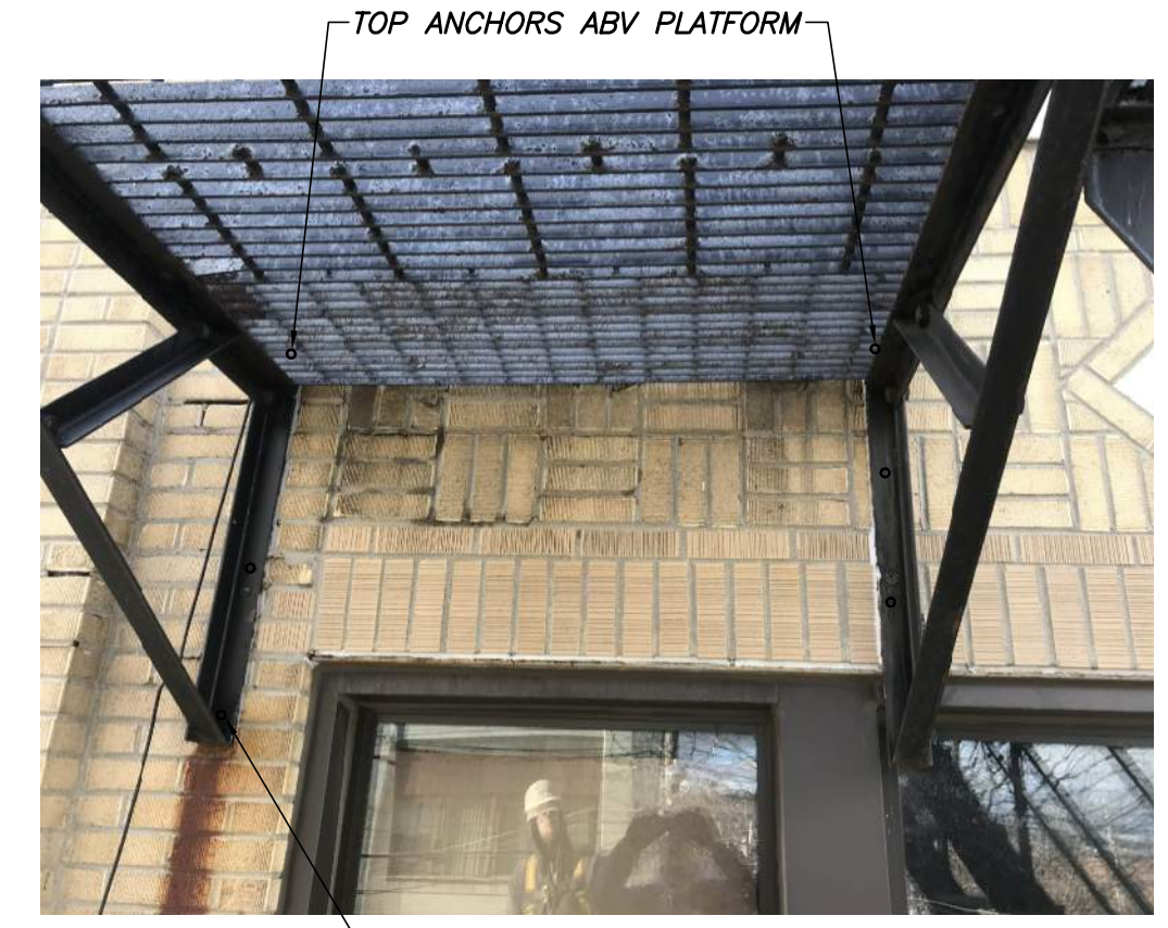
PHOTO 4 TOP ANCHORS ABV PLATFORM PROVIDE NEW ADHESIVE ANCHORS, 3 PER BRACKET (SEE GENERAL NOTES FOR ADDL INFO)
