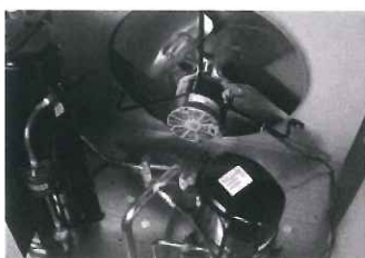
Typical Outdoor Unit with three-way liquid-line filter and sight glass
