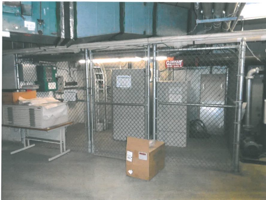
Photo 4: Sample photo showing the existing Sprint equipment.
