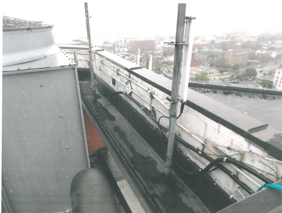
Photo 2: Sample photo showing the existing antenna.
