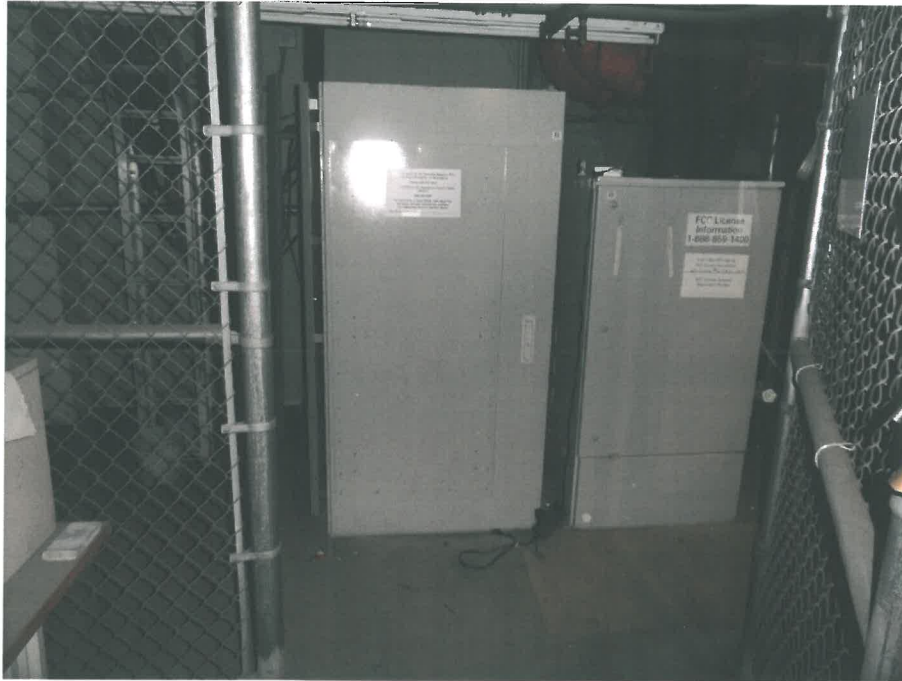
Photo 3: Sample photo showing the existing Sprint equipment.
