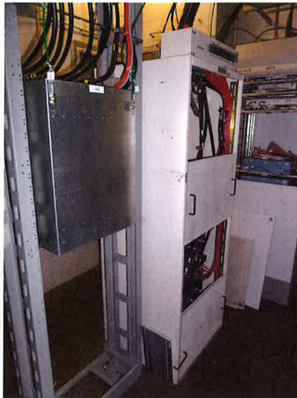
Photo 2: Sample photo illustrating the existing equipment cabinets
