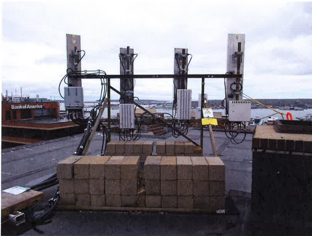
Photo 1: Sample photo illustrating the existing non-penetrating ballast mount.
