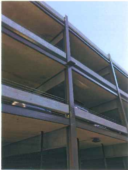
Image-03 West (Hyatt Place) facade showing garage after brick is removed, steel refurbished and galvanized automobile guard added.
