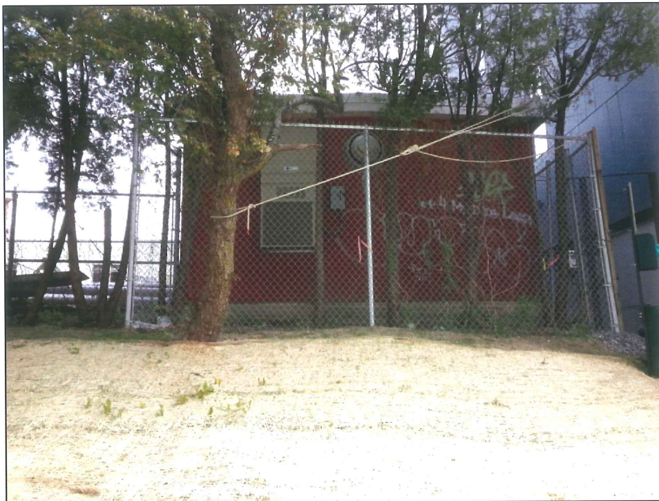
Photo 2. The tree with the rope will likely be replaced. Saplings within the fenced area and saplings immediately to the left of the fence will be removed. Note the HVAC system on the left and vandalism on the right side of the building.
