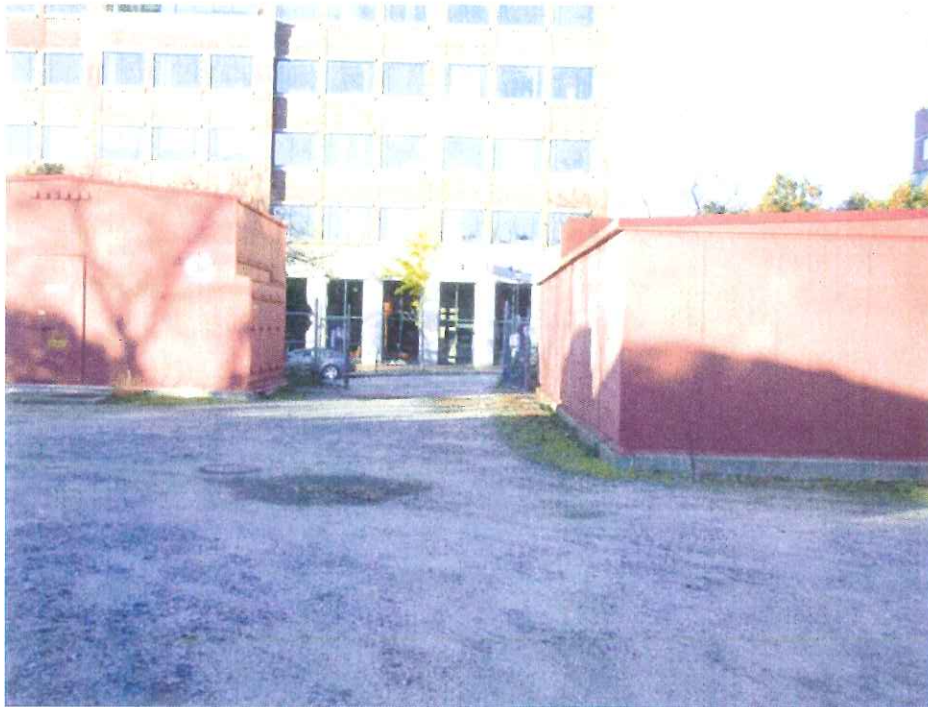
Photo 3. Existing 11.5 kV switchgear on the left to be removed. Existing 34.5 kV switchgear on the right to be replaced.
