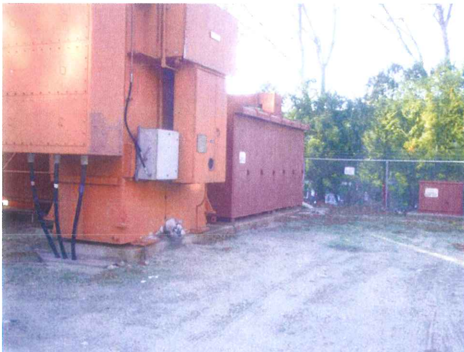
Photo 4. Existing transformer (foreground) and 12 kV switchgear. The transformer is being relocated and the switchgear is being replaced and relocated.
