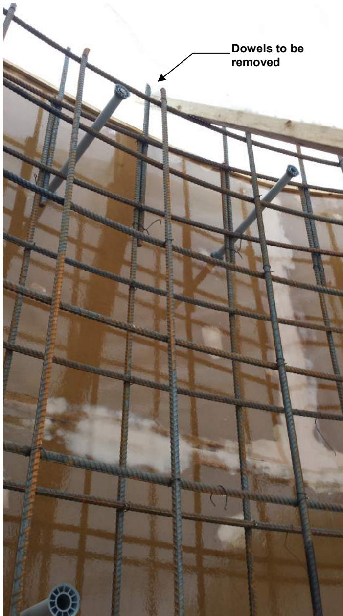
Photo 1: Vertical Dowels in the Wrong Position for Sleeve Install in Slab
