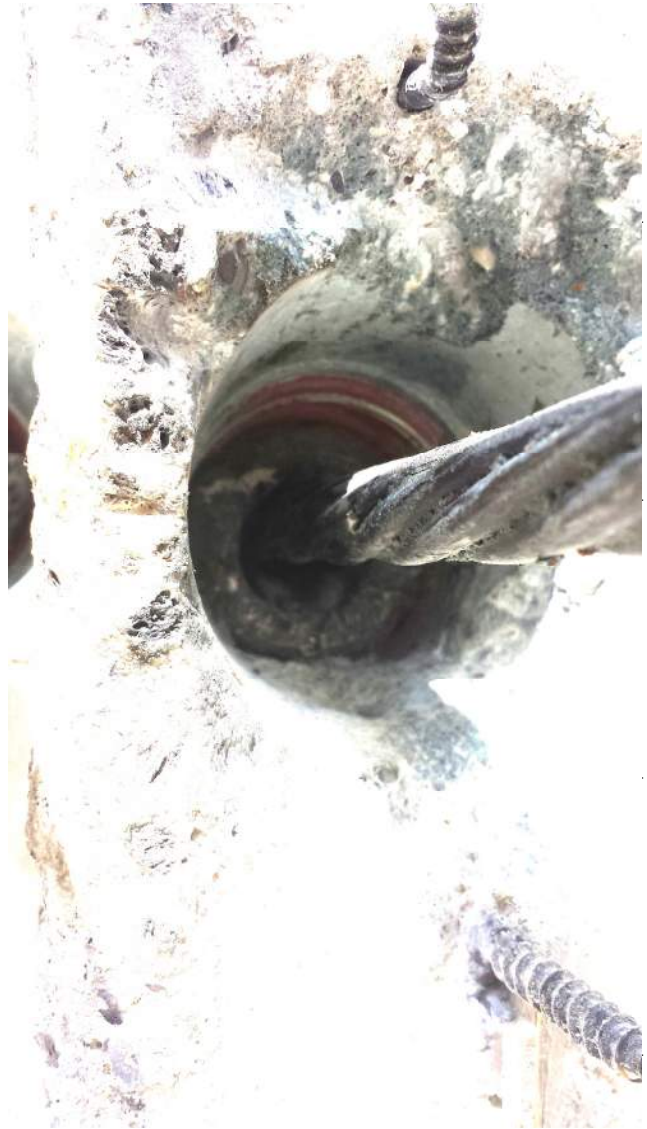
Photo 2: Concrete observed inside anchor where wedges are to be seated
