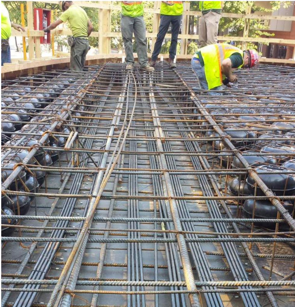
Photo 1 – “Kinked” Tendon Bundle at the end of Beam 1
