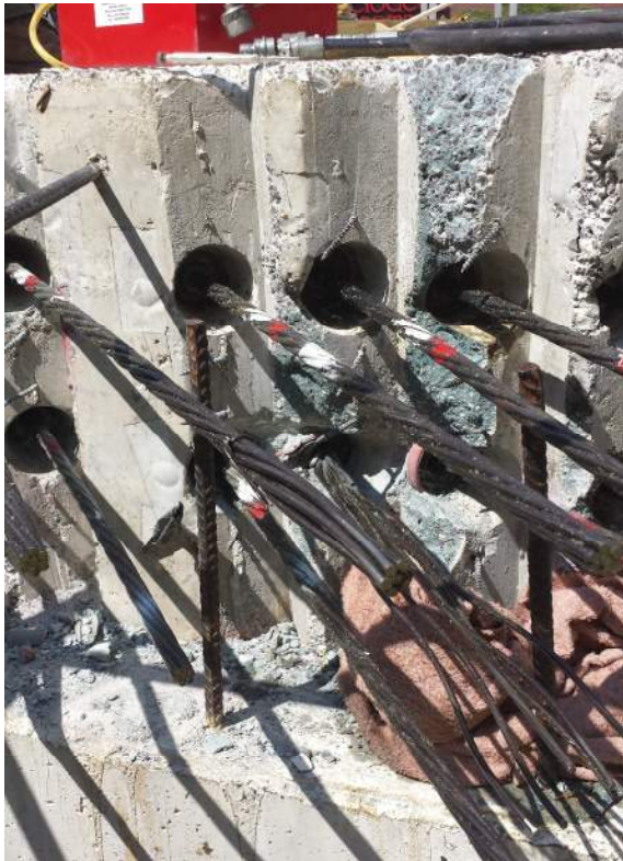
Photo 3: Broken strand at PT Beam 1
