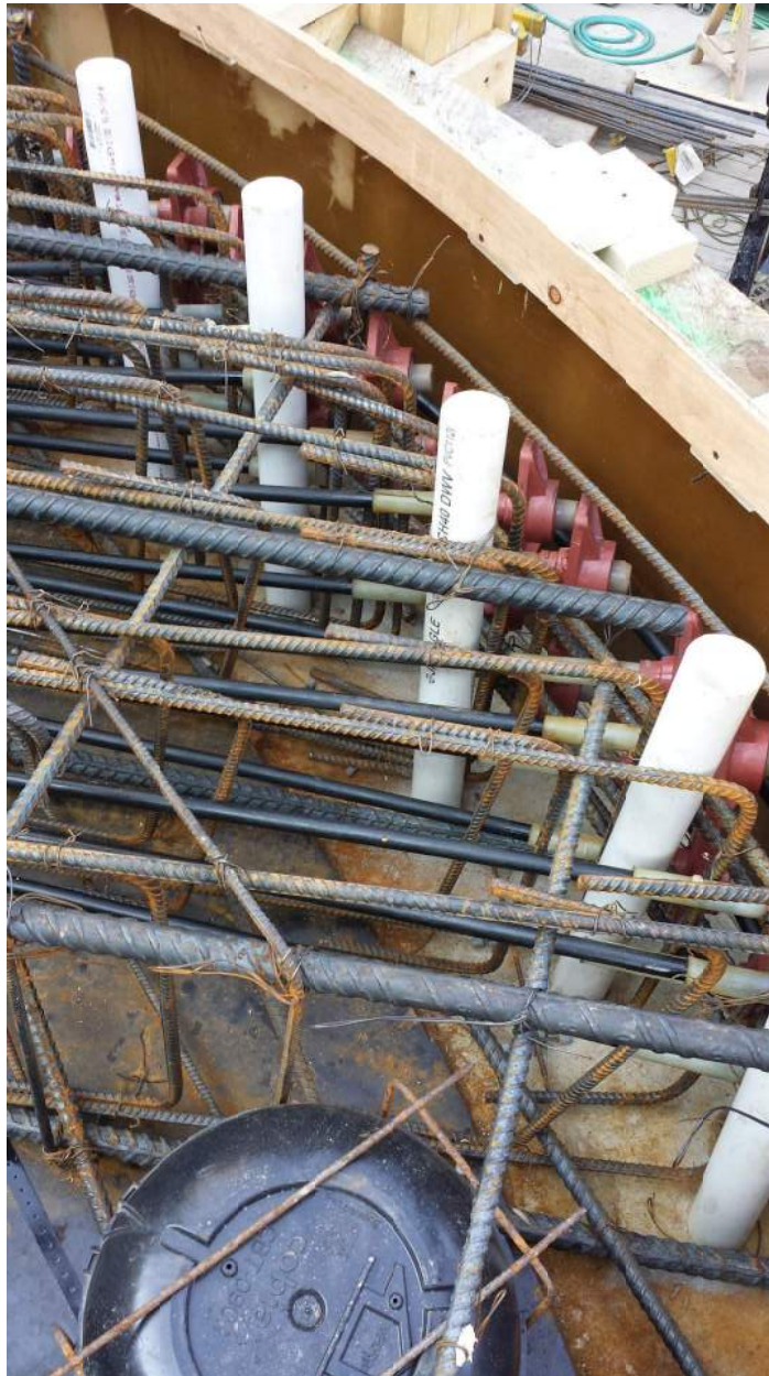
Photo 2 – Hairpins not aligned straight vertical at end of Beam 1
