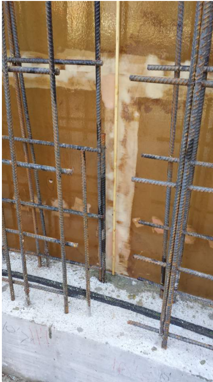
Photo 1: Vertical Control Joint w/ Horizontal Bars Cut at Both Wall Faces
