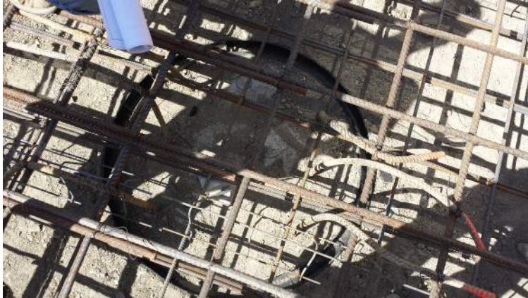
Photo 1: Damaged dowels at pier
