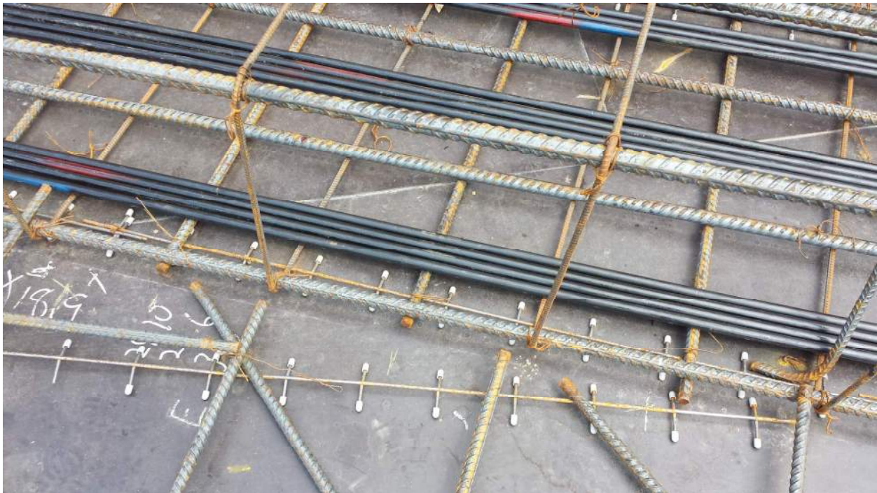
Photo 1 – Bottom Reinforcement Not Extended into Beam
