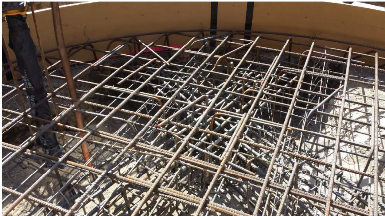
Photo 3: Grade beam horizontal bars with reversed priority (grade beam on right side should have top-most bars instead of grade beam on the left side)
