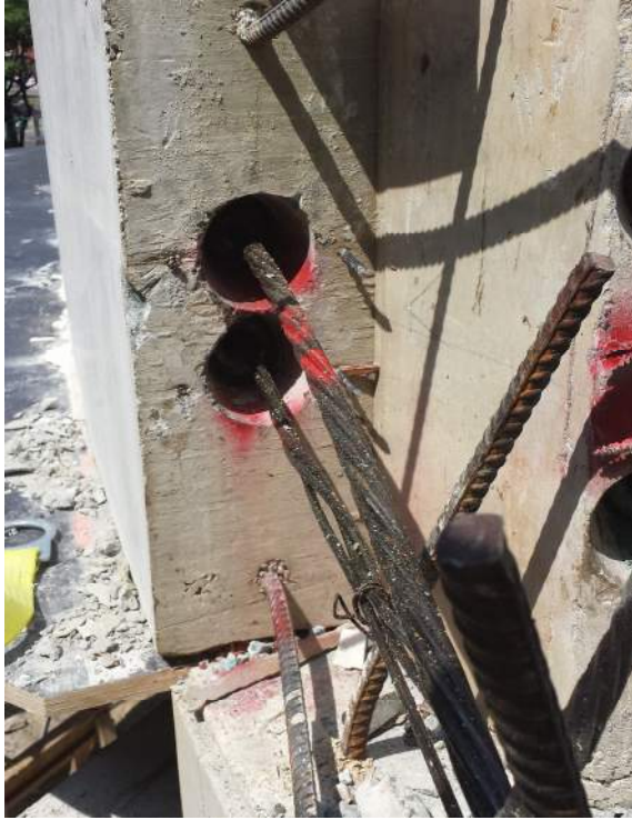
Photo 1: Broken perimeter temperature strand
