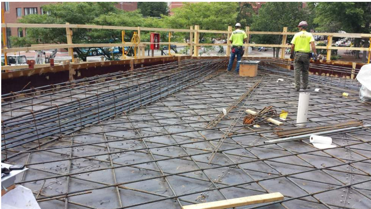
Photo 3 – PT tendons in beams not yet laid to correct profile
