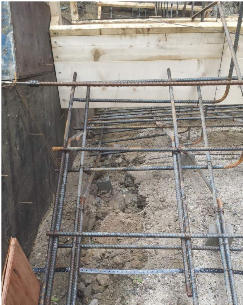
Photo 1: Washed out Grading Below Footing
