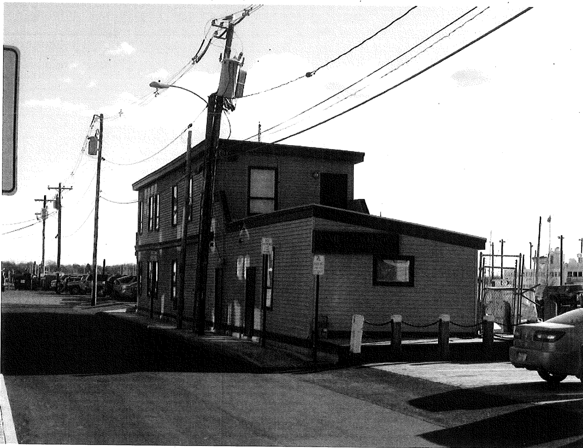
The 39 Portland Pier building is located on a pile supported timber pier. Note new road/sidewalk construction.
