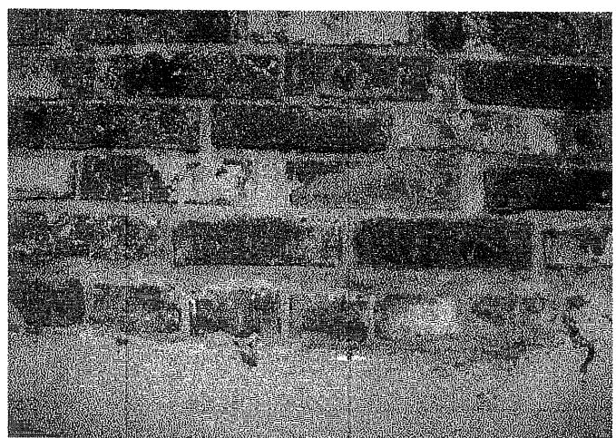
Mineral deposits on brick interior wall from water intrusion.
