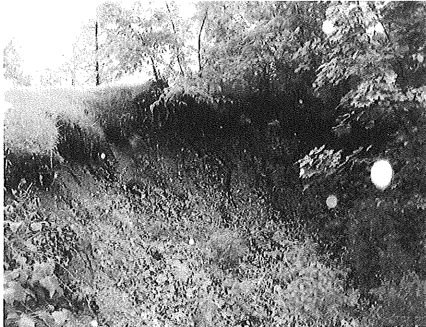
A 6'-8' high vertical face is located along the upper rim of the slide.
