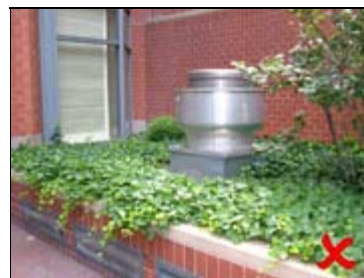
A prohibited vent structure that impairs visibility and would no longer be allowed under the current public plaza regulations
