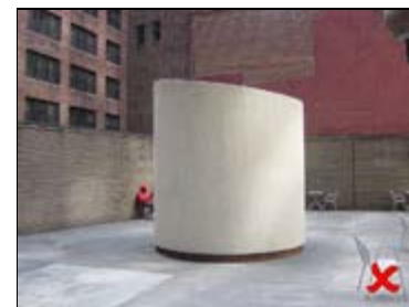
A prohibited exhaust vent that separates the plaza and would not be permitted if proposed today
